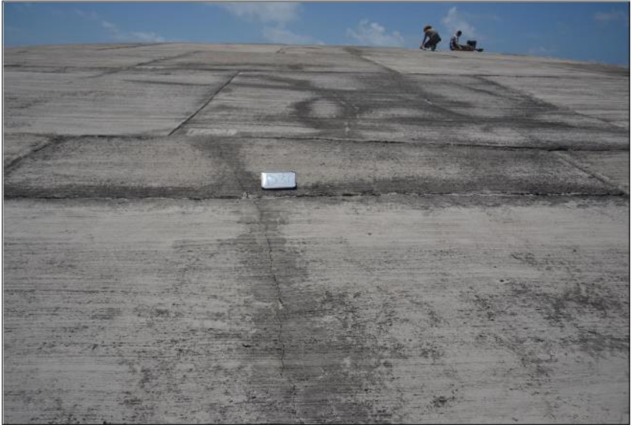
Figure C.2. Runit Dome in 2013, showing cracks and discolored concrete. Source: LLNL-TR-648143, Terry Hamilton, “A Visual Description of the Concrete Exterior of the Cactus Crater Containment Structure,” October 2013, Figure 17. This source is in the Public Domain.
