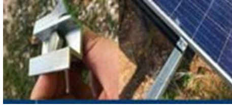
Figure 31. Top-down module clamp bent unevenly from frame deflection
