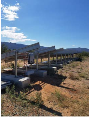
Figure 7. A ground array in Prescott, Arizona
