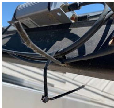
Figure77. Failed plastic wire tie
