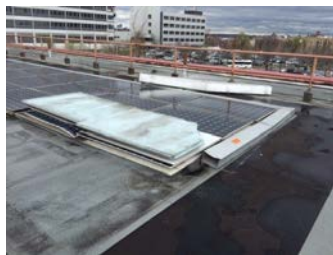
Figure 51. A severely damaged PV system in Bronx, New York
