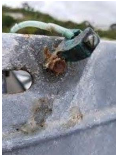
Figure 79. Corroded PV components
