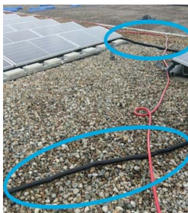
Figure 76. Exterior-rated PV wires laying across a roof
