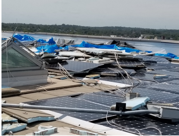
Figure 10. Ballasted array lifted off a roof surface
