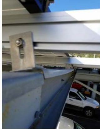
Figure 29. Bent top flange of a c-channel
