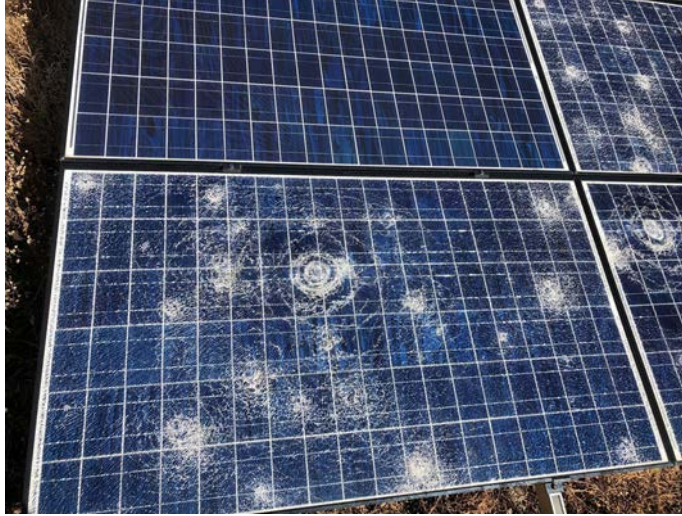
Figure 56. Breakage of one large hailstone allows smaller ones to break the glass weakened by cracks, but the PV module material stays in the frame. Photo by Andy Walker
