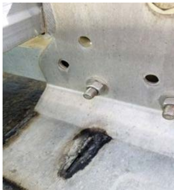
Figure 33. Vibrational loosening of a bolted joint
