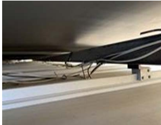
Figure 78. Failed plastic wire ties
