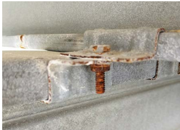
Figure 48. Corroded components from rains with high salt content
