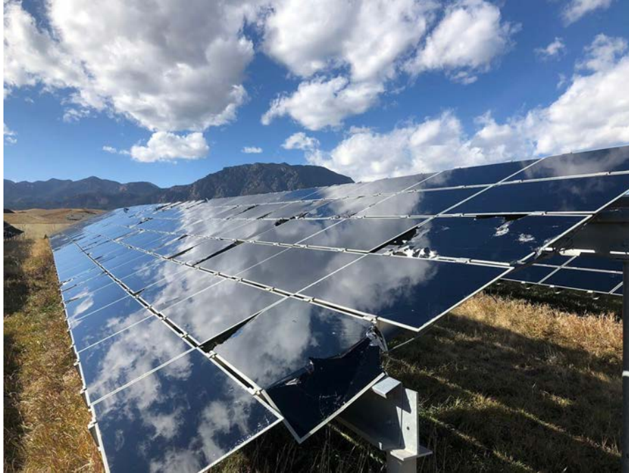
Figure 57. Hail damage to an array in Fort Carson, Colorado, caused by hailstones on the order of 2.75 cm diameter that fell on August 6, 2018.
