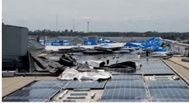
Figure 52. A severely damaged PV system in Grand Rapids, Iowa
