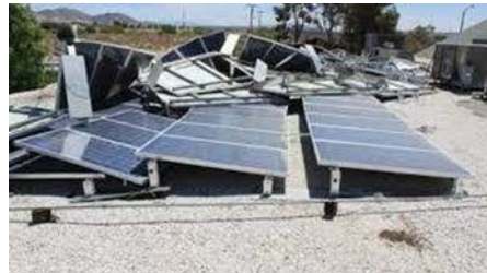
Figure 9. Ballasted rooftop array with inadequate mechanical attachment points
