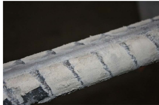
(b) concrete powder between ribs
