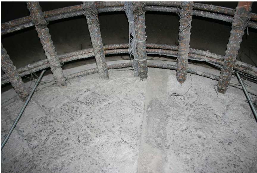
Figure B.8: Construction joint at footing-shaft interface after steel brushing (same preparation for all construction joints)
