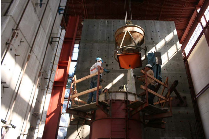
Figure B.9: Concrete pour of the lower portion of the shaft (Pour 2)
