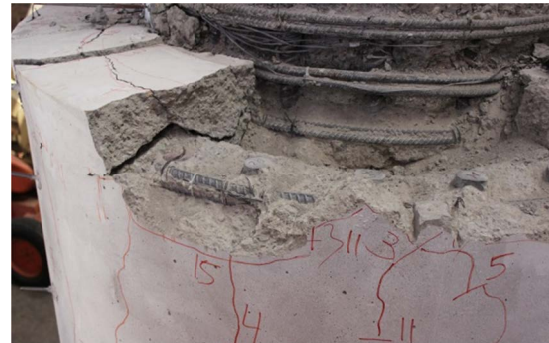
(d) Post-test inspection (Top of south face)
