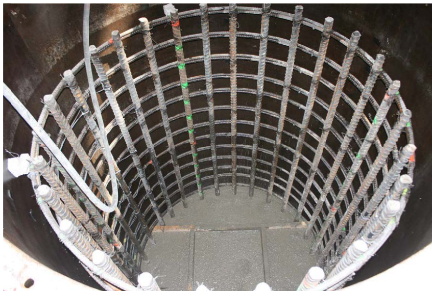
Figure B.10: Pour 2 completed at the level to which the column cage will be embedded
