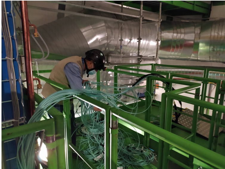
Figure 6.23: The green cables contain optical fibers coming from the GE1/1 detectors. At this point, the fibers are on top of the CMS experiment and here they are being carefully organized and coiled before being attached to a patch panel.
