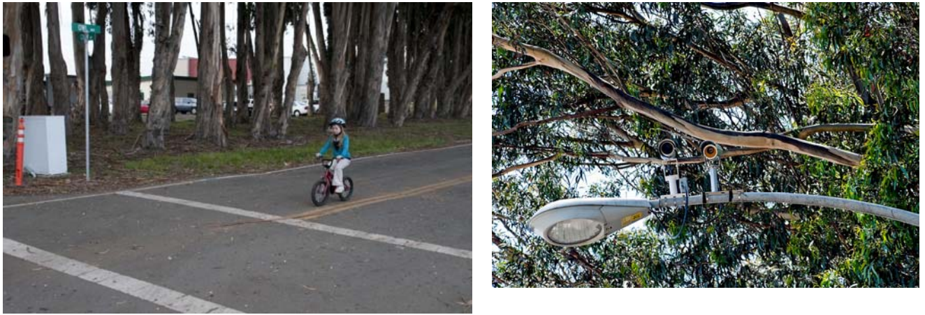
Figure 26 Nominal-Size Bicyclist (4 feet tall, 90 pounds) Riding the Test Bicycle Just Inside the Lane Boundary for Testing Video Detection System, Using Traficon Camera Mounted on Mast Arm (right in right photo)
