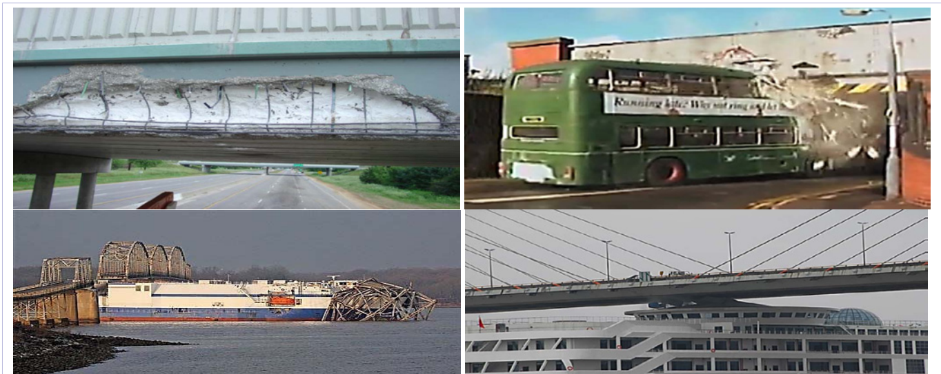
Figure 13: Impact damages in the concrete bridge girders by over-height trucks and buses.
