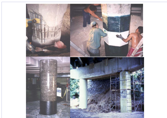
Figure 1: Repair and rehabilitation of corroded bridge & buildings RC columns with FRP composites.
