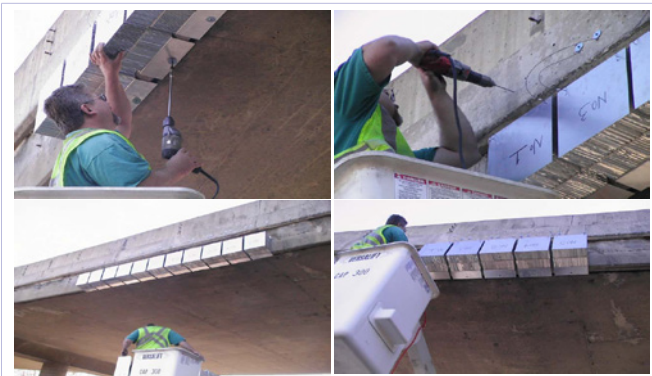
Figure 16: First field application of the I-Lam over height collision protection System in Ohio, USA.
