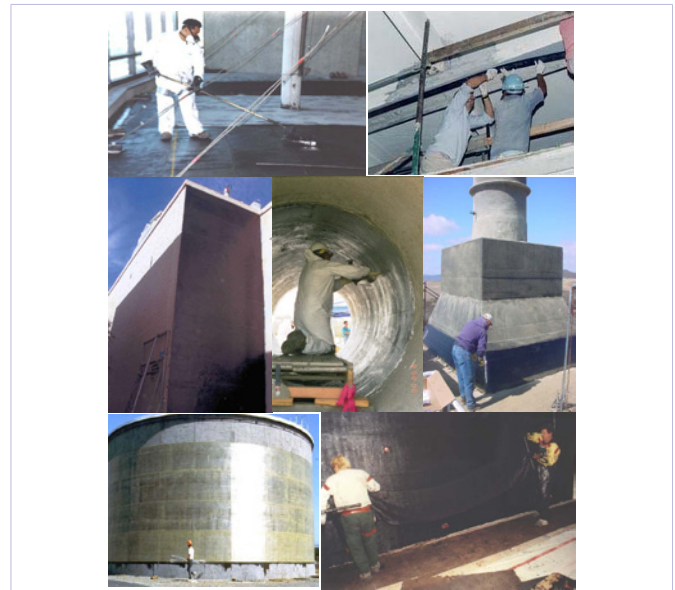
Figure 2: Examples of strengthening applications of FRP composites. a. Floor beams; b. Floor slabs; c. Masonry walls; d. Pipes; e. Foundations; f. Tanks; g. RC Shear walls
