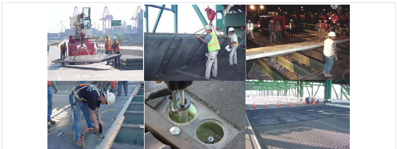
Figure 36: Field installation of the hybrid composite bridge deck at the Schuyler Heim bridge site, Long Beach, California, USA.
