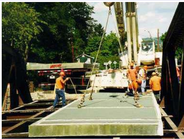
Figure 37: Installation of all-composite bridge deck of NY 367 over Bentley Creek, Chemung County, New York, USA.
