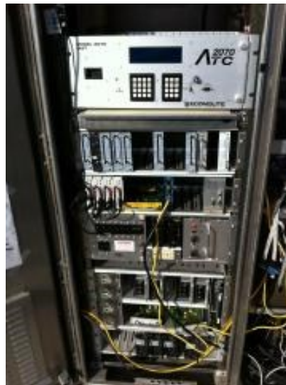
Fig.5.4. Traffic Signal Controller
