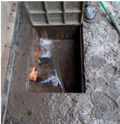
5) Formal sewer at public toilet (usually covered)
