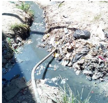
Figure 7: ‘Spaghetti’ Water Pipe Passing through Open Drain and Solid Waste
