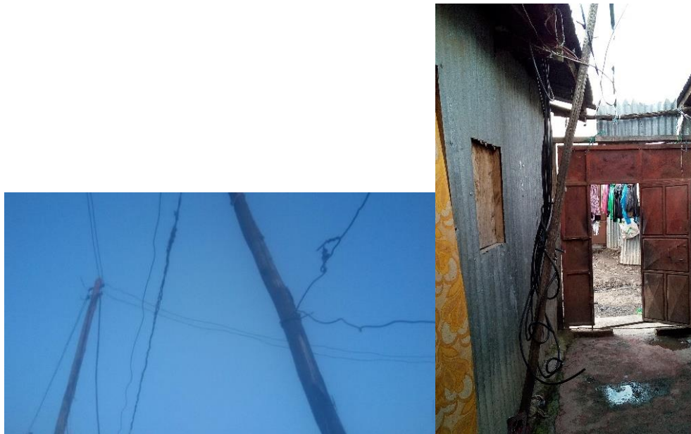
Figure 3: Multiple Types of Informal Electricity Wiring in Mukuru
