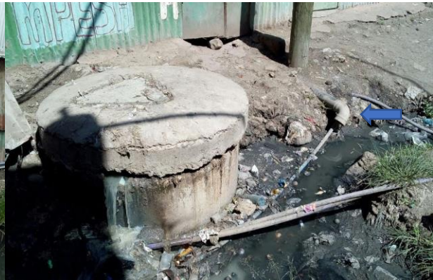
4) Overflowing manhole (near pipe to drainage)
