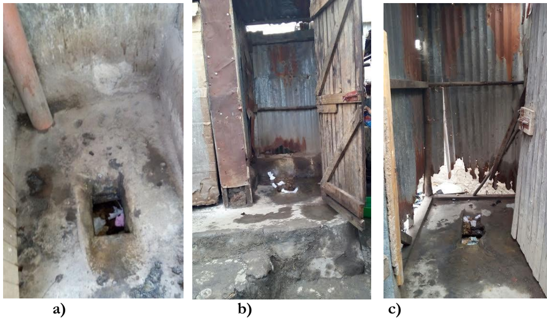
Figure 3: Typical Latrines in Mukuru a) Ventilated latrine (see pipe in upper left) not yet full but with menstrual waste; b) latrine with raised structure and overflowing solid waste; c) nearly-full latrine with rusted sheets
