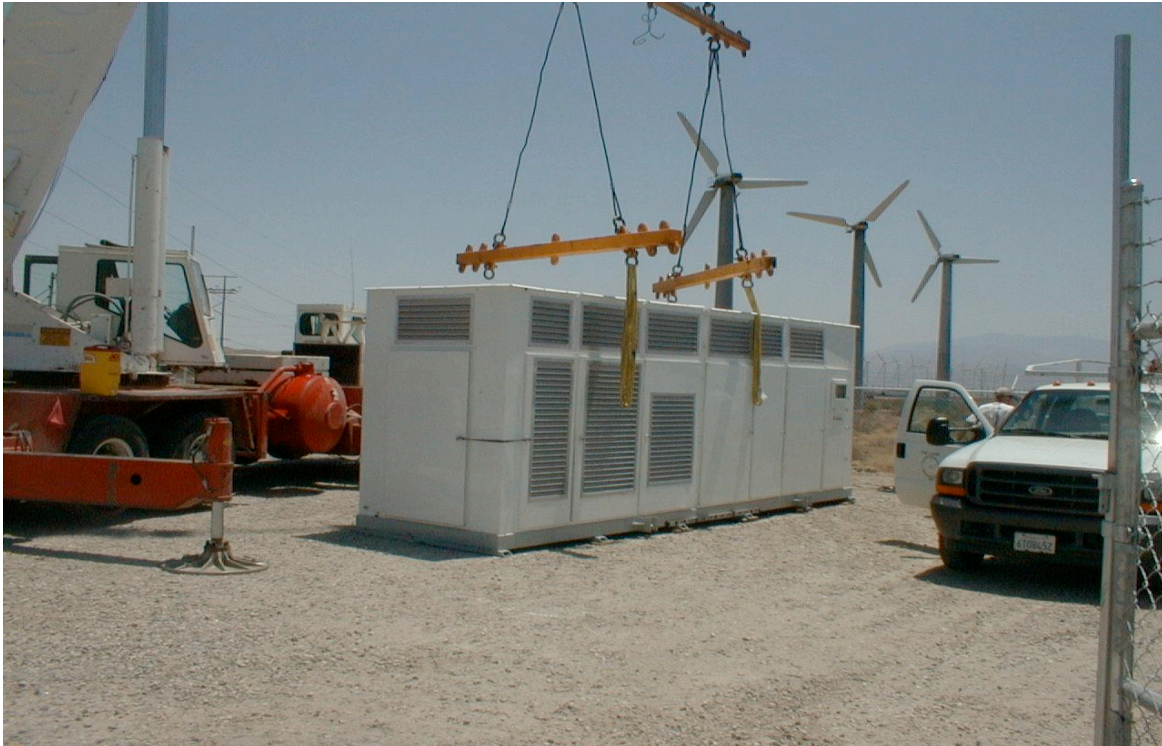
Figure 7: Hydrogen Electrolyzer System Being Installed Near Wind Farm in Palm Springs, California
