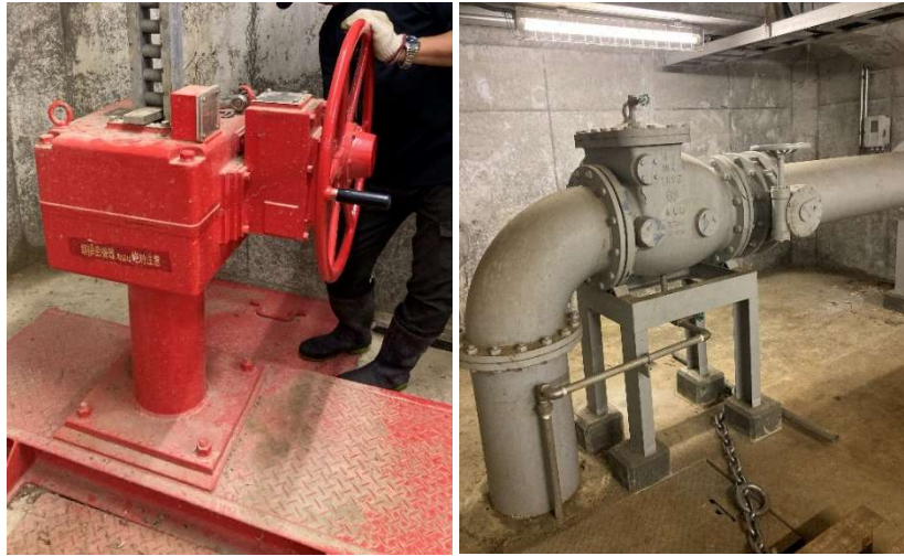
Image: Equipment at the Nibutani Dam's pump house.
