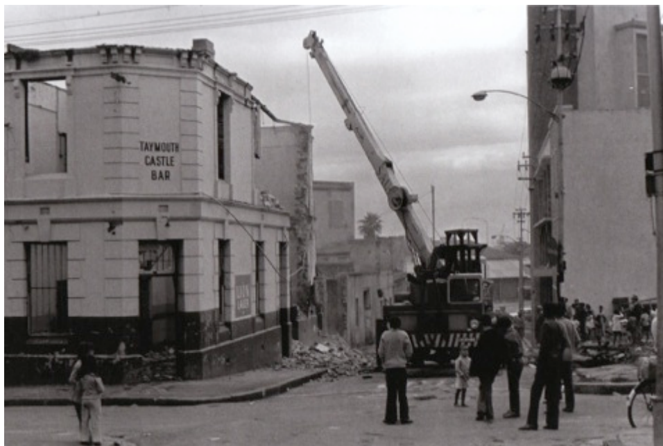
Figure 3.5 Demolition. District Six was bulldozed, building-by-building and street-by-street to produce the city in the image of apartheid governmentality. From Hallett 2007, 107.
