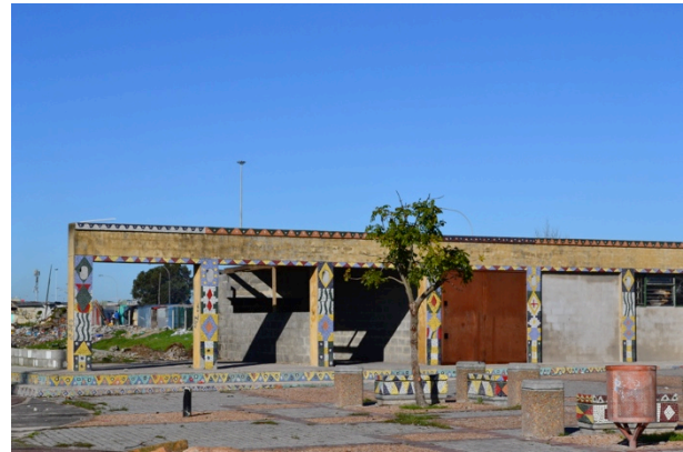
Figure 4.17 Philippi Plaza Trading Frame. The mosaic-decorated concrete frame, intended for attaching trading stalls, remains unused. Photo by author, 2013.
