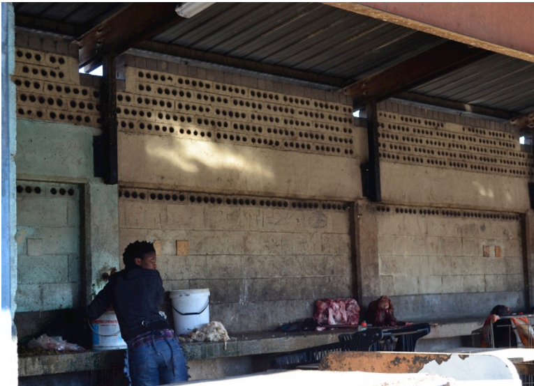
Figure 4.31 Ventilation Blocks. The blocks installed at the upper portion of the walls of the meat selling buildings are perforated with holes to allow light and ventilation. Photo by author, 2012.
