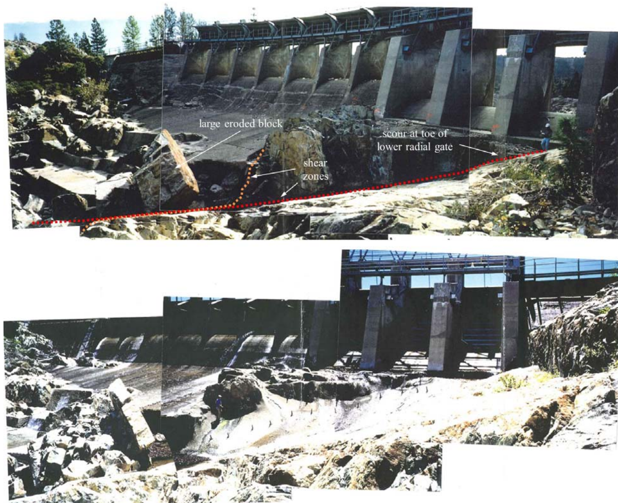
Figure 3-9. Scour (top) and remediation (bottom) downstream of three lower radial gates (Page 1997, 1998). Note person for scale.
