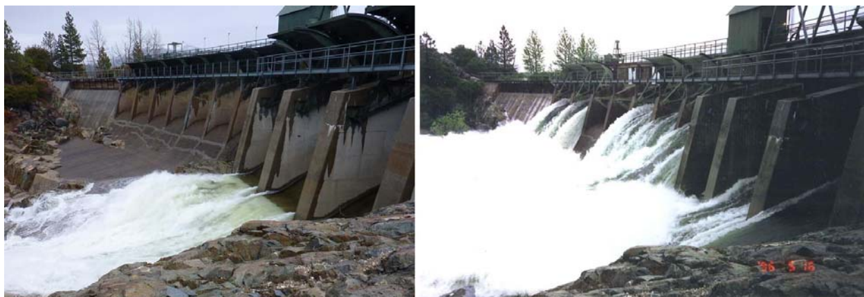
Figure 3-5. Dam No. 2 current geometry (left, December 2012 spill event approximately 14 \text{m}^3/\text{s} ) and May 1996 spill event (right, 716 \text{m}^3/\text{s} , photo from Mattson (1996)).
