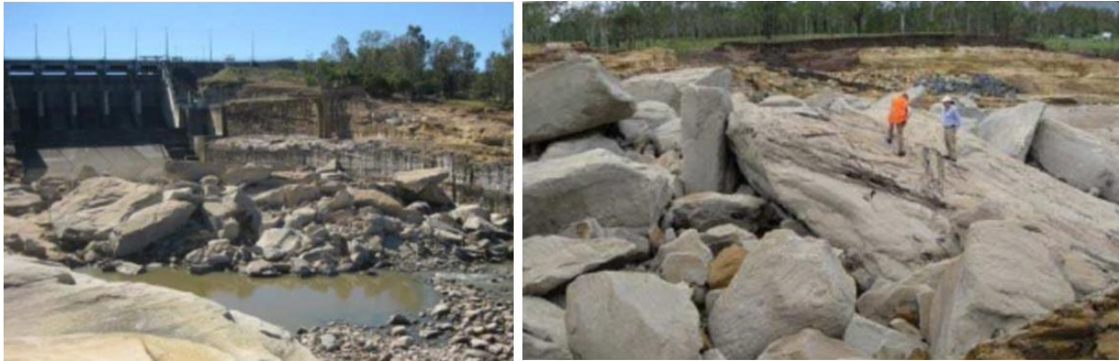
Figure 1-2. Removal of large rock blocks from unlined spillway at Wivenhoe Dam in Australia (Stratford et al. 2013). For scale, spillway width is approximately 90 m.
