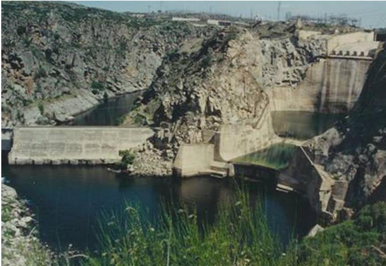
Figure 1-5. Scour remediation at Ricobayo (note extensive excavation and concrete work in the plunge pool region in addition to flow splitters on the spillway lip to dissipate hydraulic energy) (photo source unknown).
