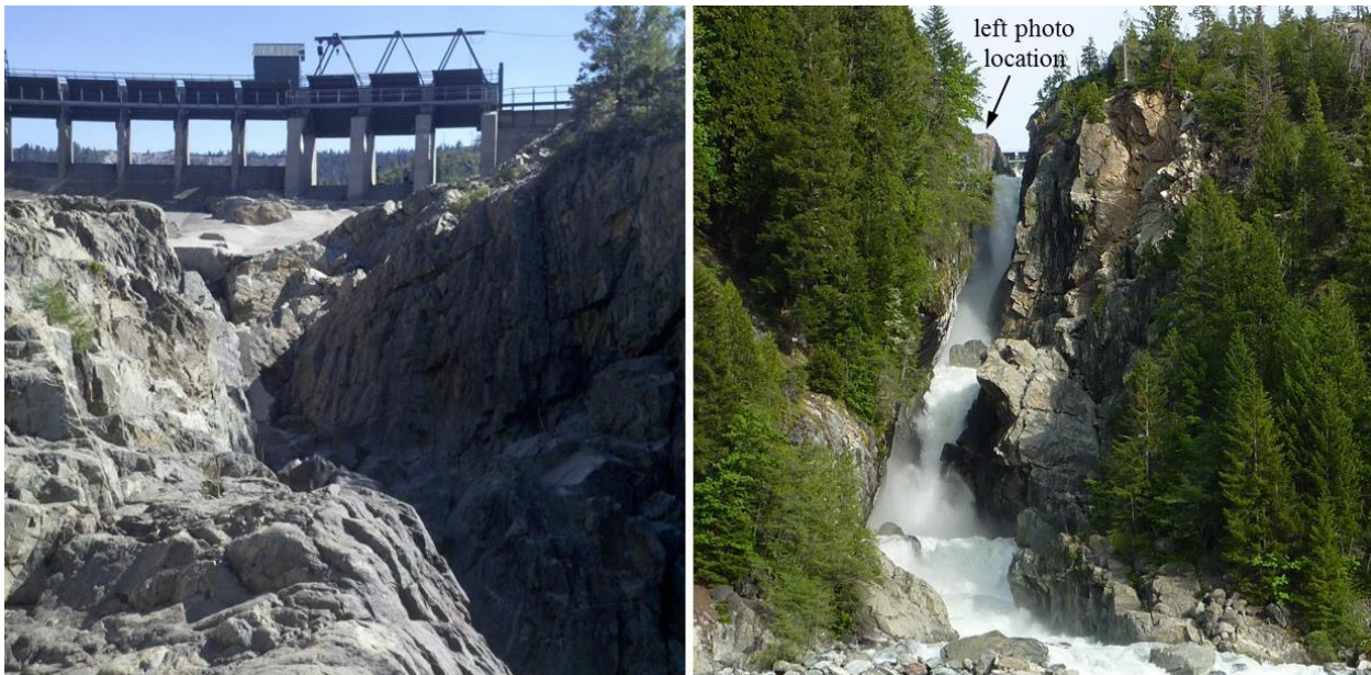
Figure 3-7. Upper reach of eroded slot canyon viewed from middle of spillway (left) and lower reach of slot canyon viewed from Jordan Creek with alluvial fan of scoured material in the foreground (right).
