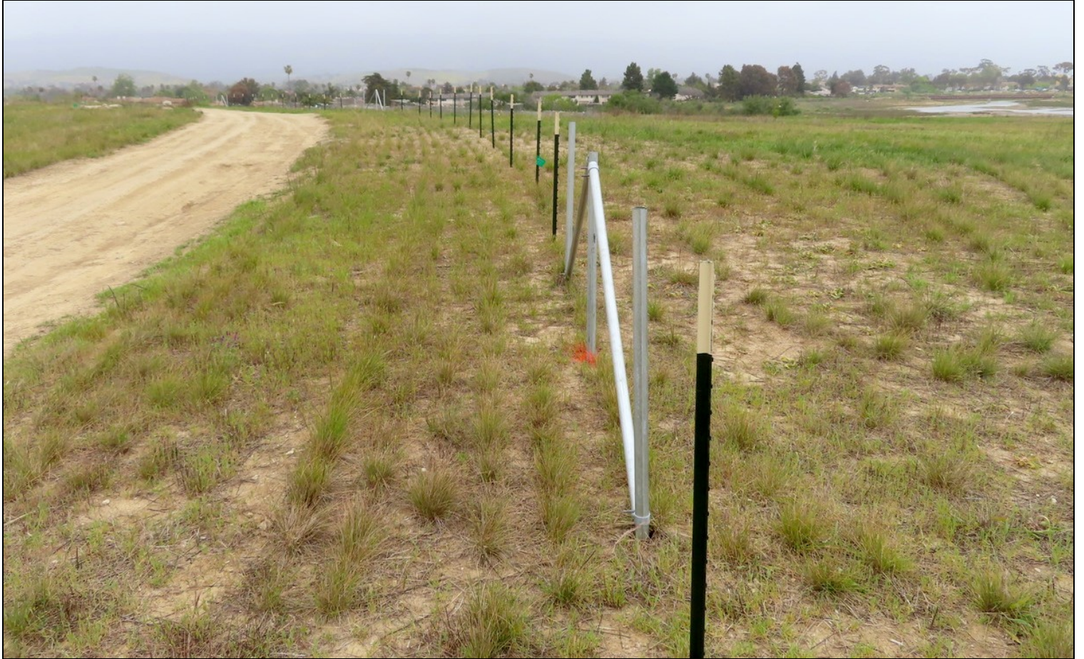
A view of the new fence being installed along the Mesa trail.
