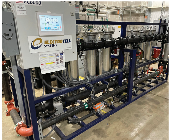
ElectroCell system installed at Toyota Motor Manufacturing, Mississippi plant. Photo from Energy 350
