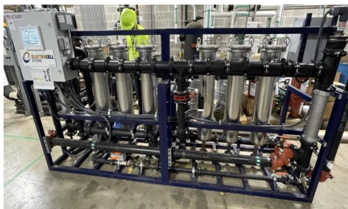
Figure 2. ElectroCell Systems Model EC-6000 installed at TMMMS
