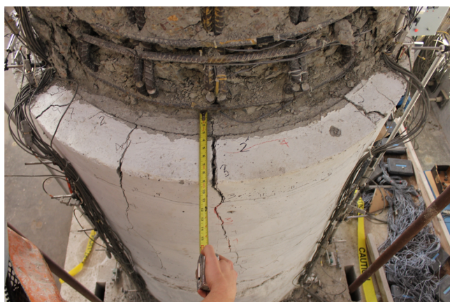
Fig. 10. Cracks atop of the pile of Specimen 4
