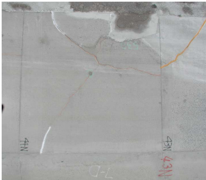
Appendix B. Figure 13. Slab 44 after DBR and HVS testing.
