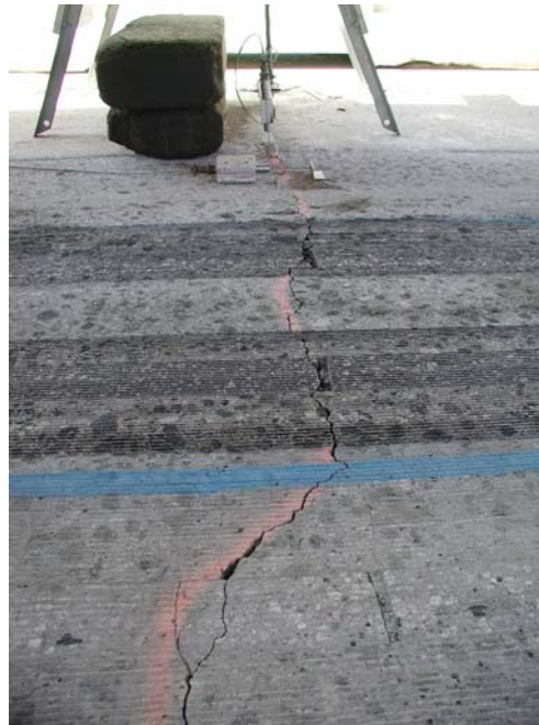
Figure 6.54. HVS Test Section 558FD, Crack 2 after 2.002 million repetitions.
