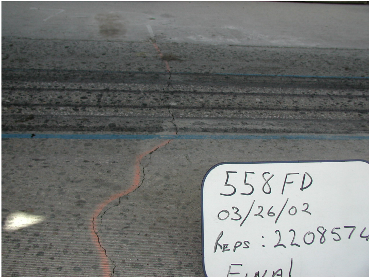
Figure 6.75. Close-up of final condition of Crack 2 at end of HVS loading after 2.209 million repetitions.
