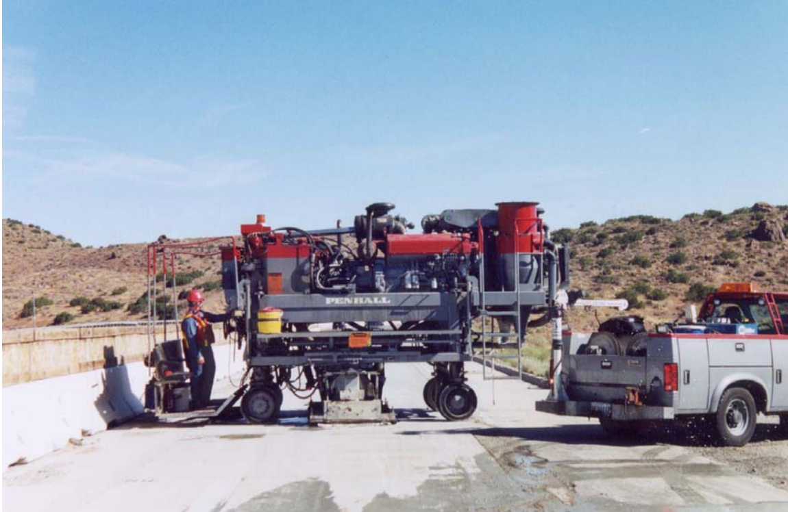
Figure 2.8. Dowel bar slot cutting machine (side view, blade arbor and vacuum between front and back wheels).
