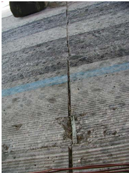
Figure 6.53. HVS Test Section 558FD, Joint 41 after 2.002 million repetitions.
