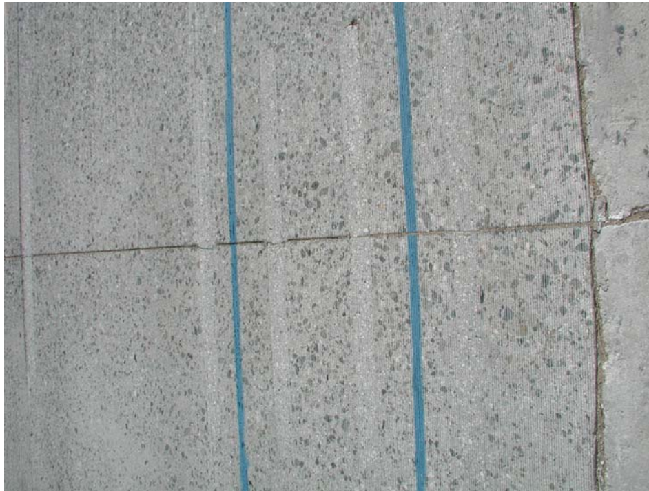
Figure 2.34. Photograph of Joint 38, Section 556FD, in March 2002, showing generally good condition. (Blue line painted on surface shows HVS wheelpath).
