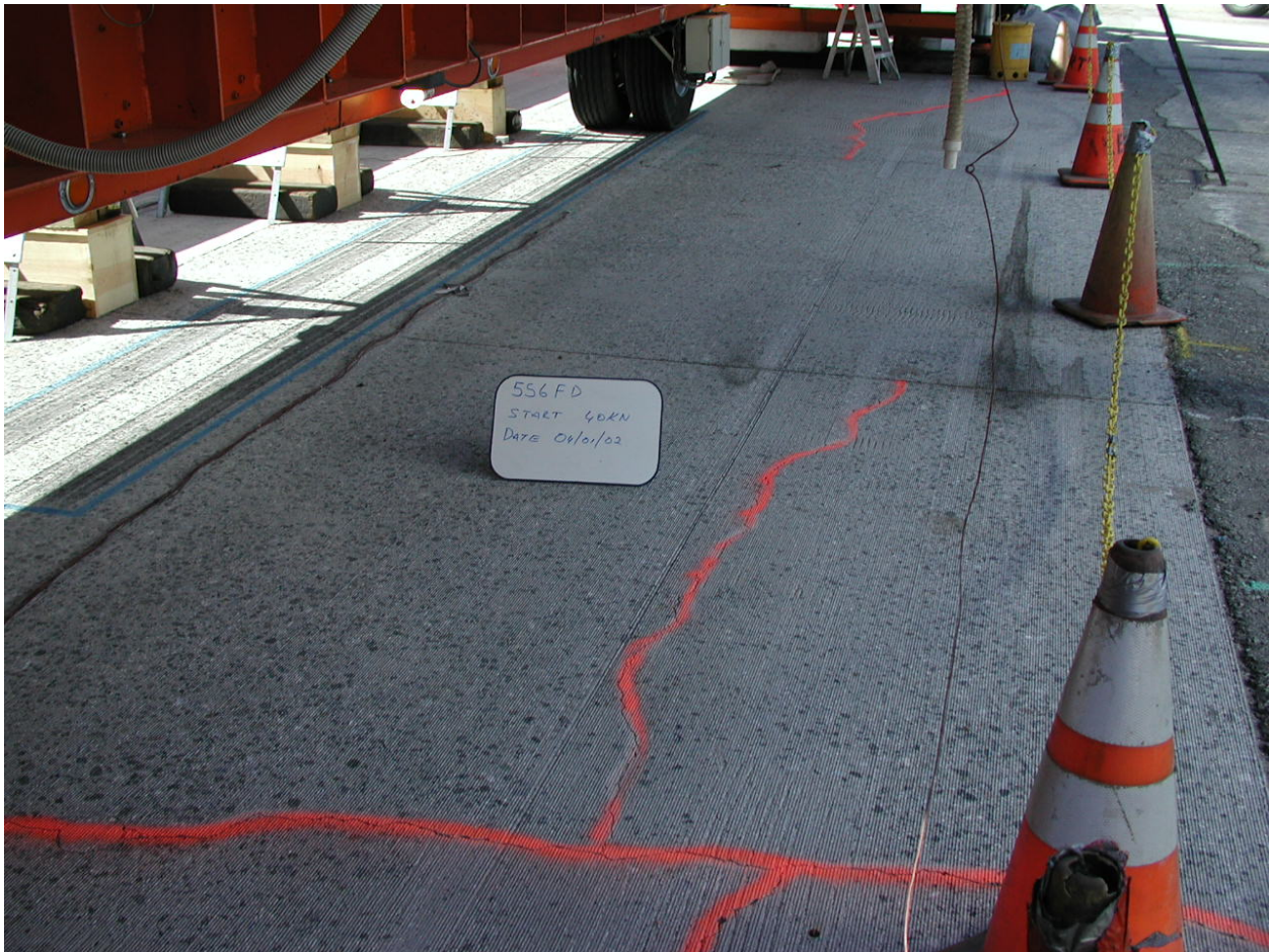
Figure 6.21. Initial condition of slabs in Section 556FD with existing cracking in adjacent slabs marked in red.
