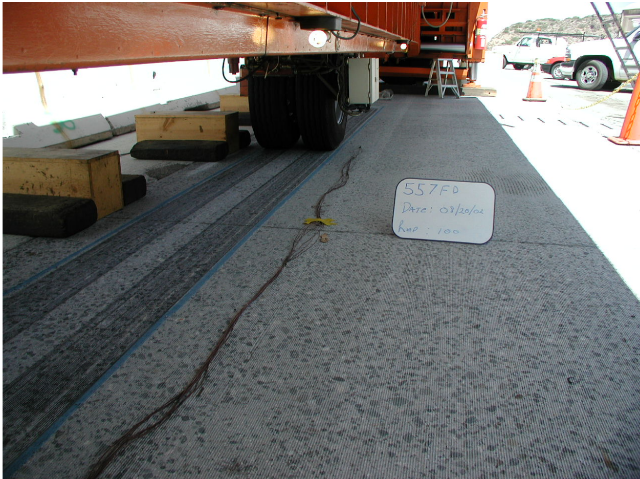
Figure 6.46. Initial condition of slabs in Section 557FD showing no existing cracking.
