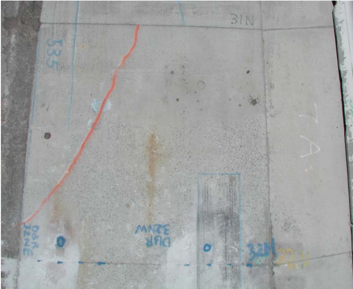
Appendix B. Figure 1. Slab 32 after DBR and HVS testing.
