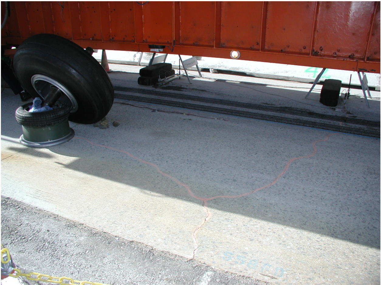
Figure 6.50. Slab 42 near Joint 41 on Section 558FD after 2.002 million repetitions.
