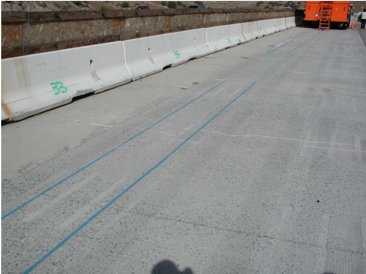
Figure 6.76. HVS Test wection 559FD prior to HVS testing. Blue lines painted on surface show future HVS wheeltrack.
