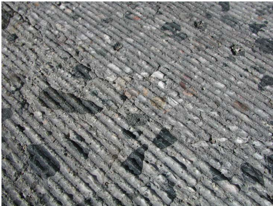
Figure 2.38. Photograph of DBR slot, Section 557FD, in June 2003, showing tight transverse cracks in grout and slab.
