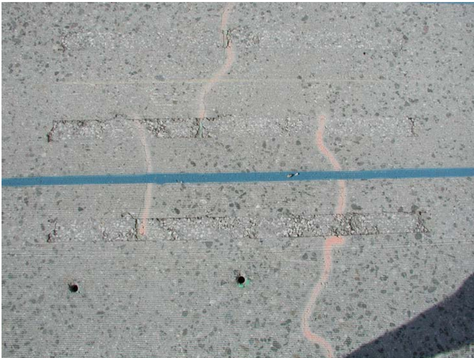
Figure 2.36. Photograph of Crack 1, Section 559FD, in March 2002, showing lack of fines, transverse cracking, and separation at edges.
