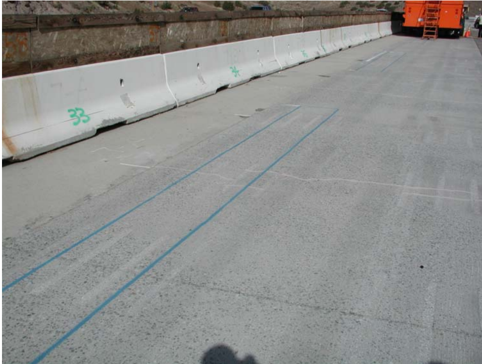
Figure 2.25. Sections 559FD (Slabs 32, 33, and 34 in foreground), 557FD (background), and 556FD (far background under front of HVS) after dowel bar retrofit and grinding, and before HVS testing.
