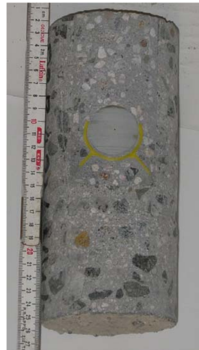
Figure 2.33. Core DBR42NNW with FRP dowel located 23 mm above mid-depth of slab.
