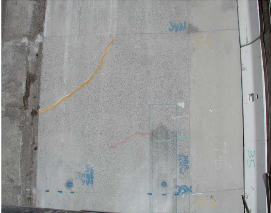
Appendix B. Figure 4. Slab 35 after DBR and HVS testing.
