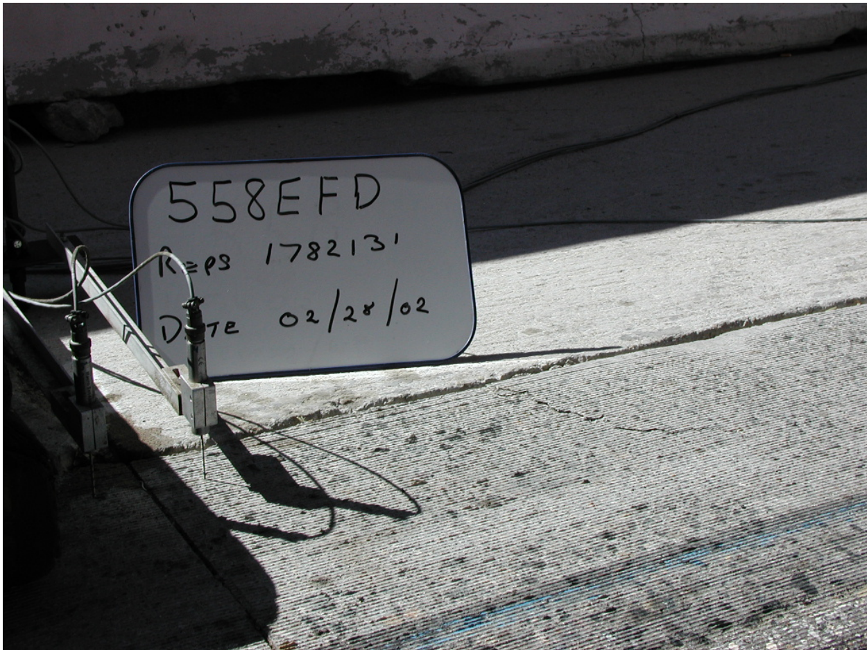
Figure 6.71. First new crack on Section 558FD from slab edge to back of outside dowel bar slot on Joint 41 at 1.782 million load repetitions.
