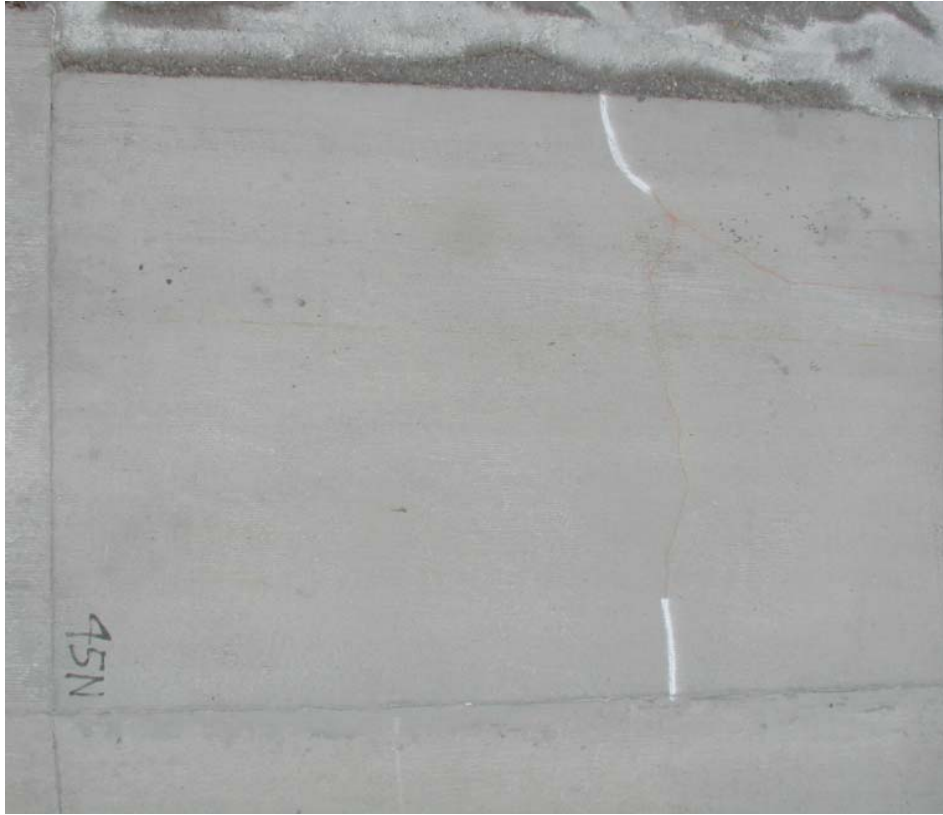
Appendix B. Figure 14. Slab 45 after DBR and HVS testing.
