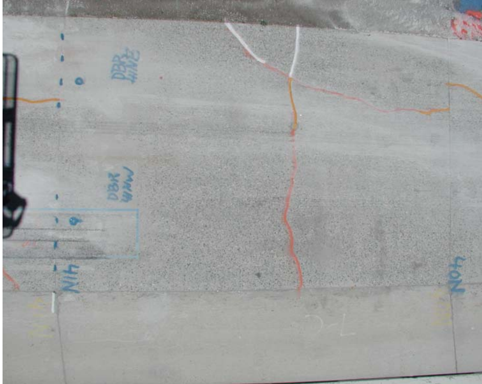
Appendix B. Figure 10. Slab 41 after DBR and HVS testing.
