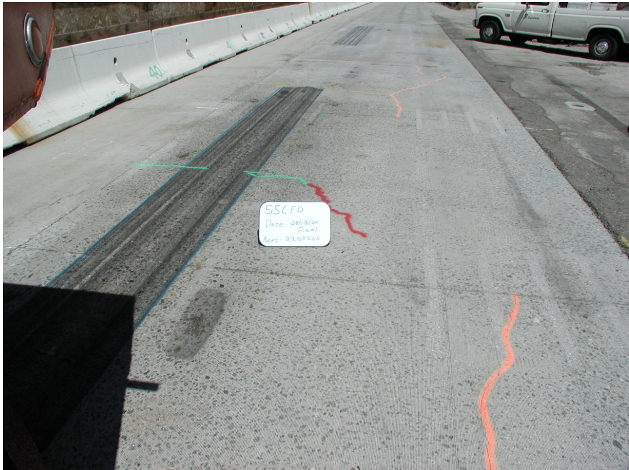
Figure 6.25. Cracking in all slabs at end of HVS loading on Section 556FD after 2.209 million repetitions.
