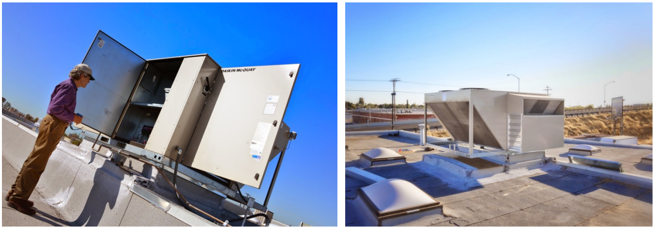
FIGURE 5: PHOTOS OF DAIKIN REBEL ON ROOFTOP
