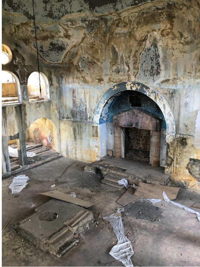
Figure 2. The ruined interior of Bhamdoun Synagogue as seen from the upstairs women's section. Image by author. September 10, 2019.
