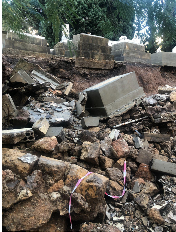
Figure 18. The aftermath of the collapse of an external wall of the Beirut Jewish Cemetery. December 27, 2019. Photo by author.
