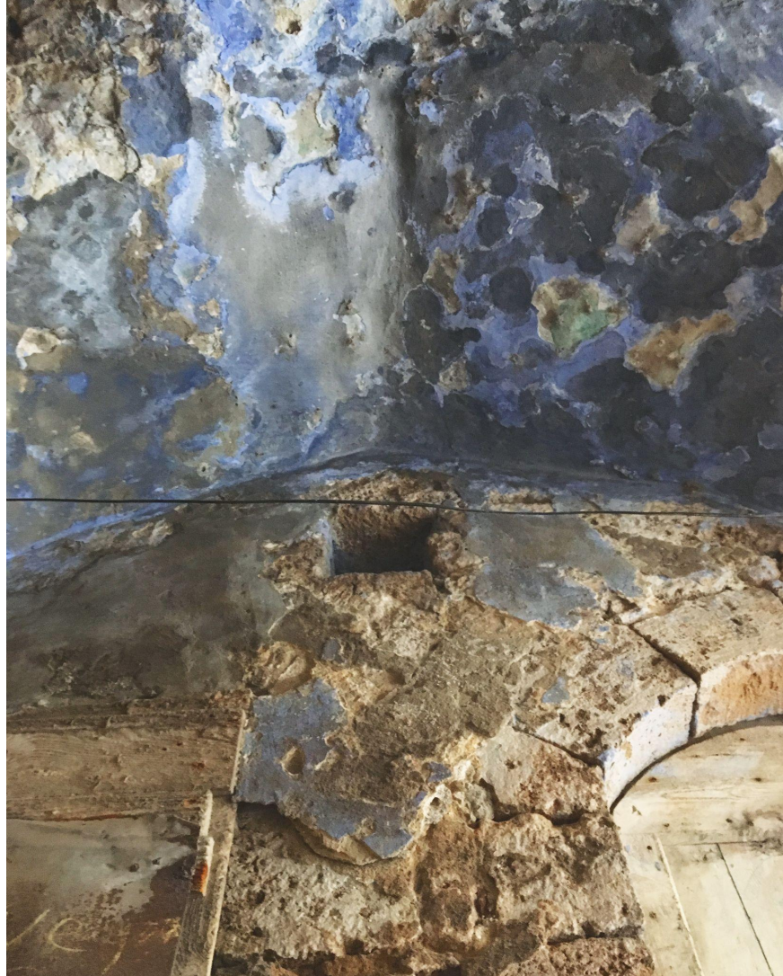
Figure 38. Blue paint, which once adorned the synagogue and its exterior, peels from the domed ceiling's stone at the structure's entrance. Photo by author. June 2018.
