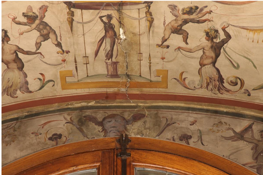
Figure 7.1 Image showing an example of the observed cracking in the Room of the Elements.
