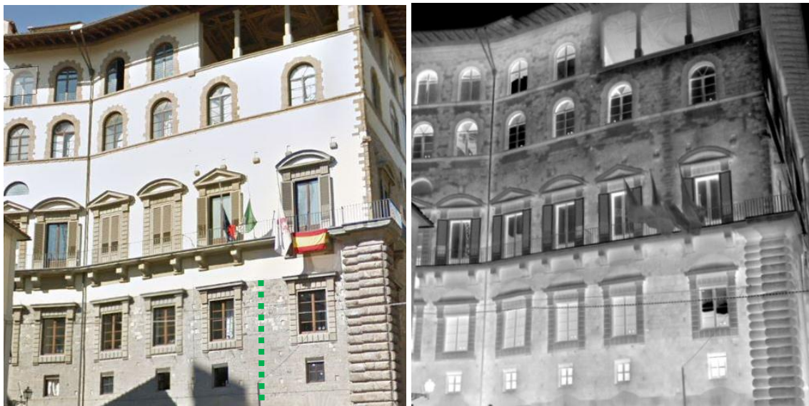
Figure 7.13 Visible and thermal layers of the South wall revealing construction details below the plaster on higher floors.
