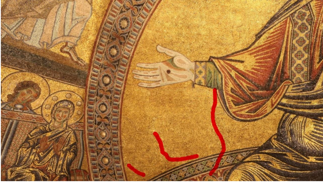
Figure 7.9 High-resolution SfM point cloud used to map the cracks in the dome through interactive annotation which highlights the cracked areas in red.
