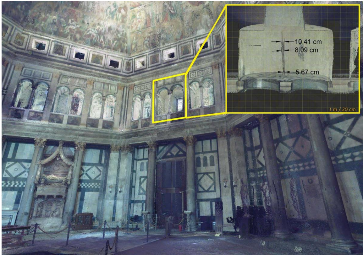
Figure 3.11 Scanning data highlighting the dimensions of a crack above the North door.
