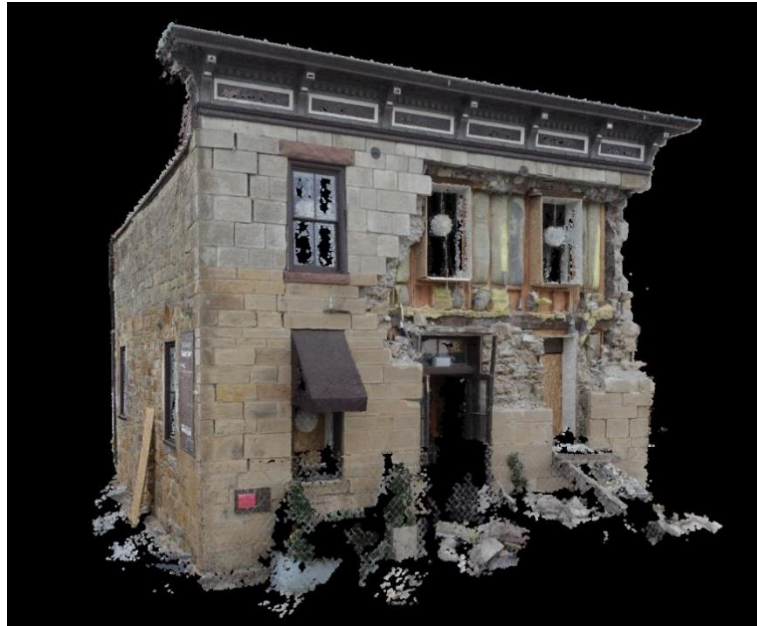
Figure 3.18 Photogrammetric point cloud of a damaged masonry structure.
