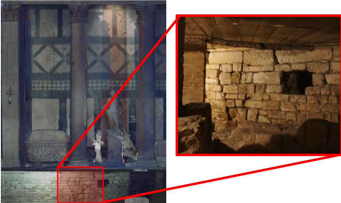
Figure 7.14 View of the foundation wall in its context with the information model (left) and an image from the excavated area showing a view of the cracked wall.
