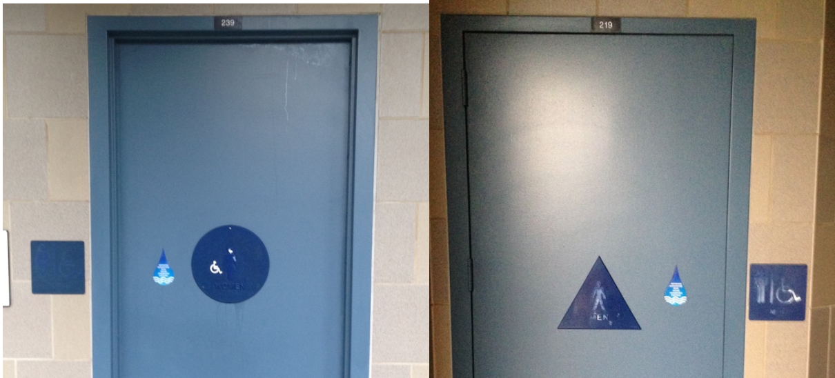
Figure 7: Defaced bathroom signs on the Humanities Instruction Building at UCI.
