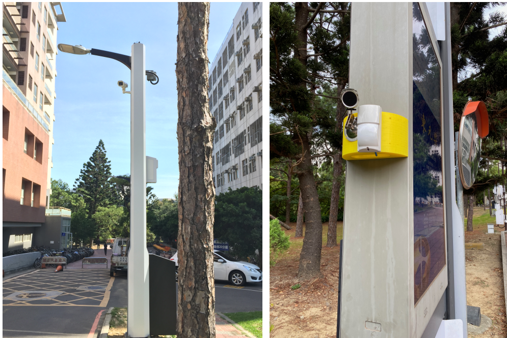
Figure 5.10: Sensor-rich smart street lamps (left) and a motion sensor (right).
