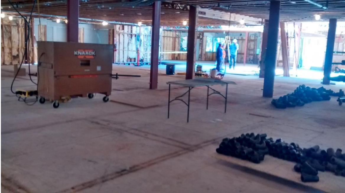
Figure 7-6 – Plumbing work start on first floor (see plumbing material, half of which is on a rolling plank)
