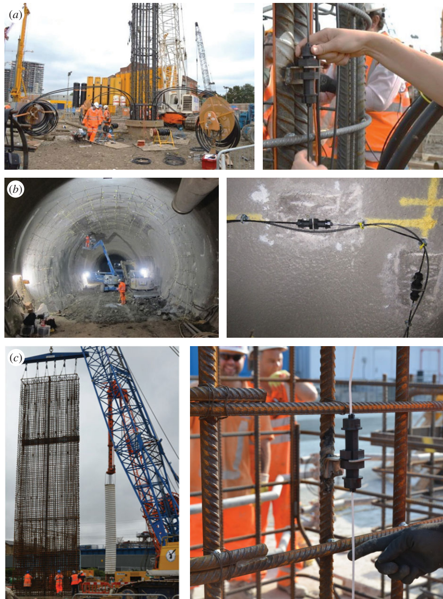
Figure 6. Examples of fibre-optics (FO) strain measurement in geotechnical structures by Cambridge University and CSIC; (a) piles, (b) tunnels and (c) diaphragm walls for underground openings. (Online version in colour.)
