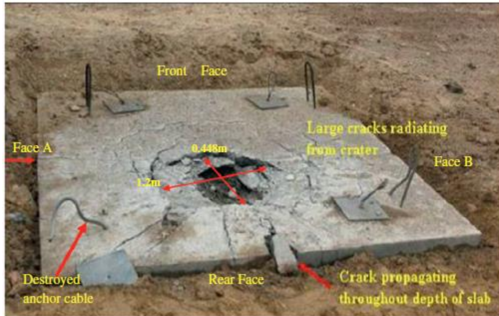
Figure 85. The crater of concrete pavement slab after blast loading [174].
