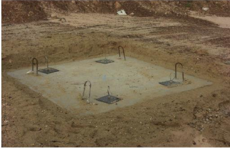
Figure 92. Concrete pavement slab before blast event [174].
