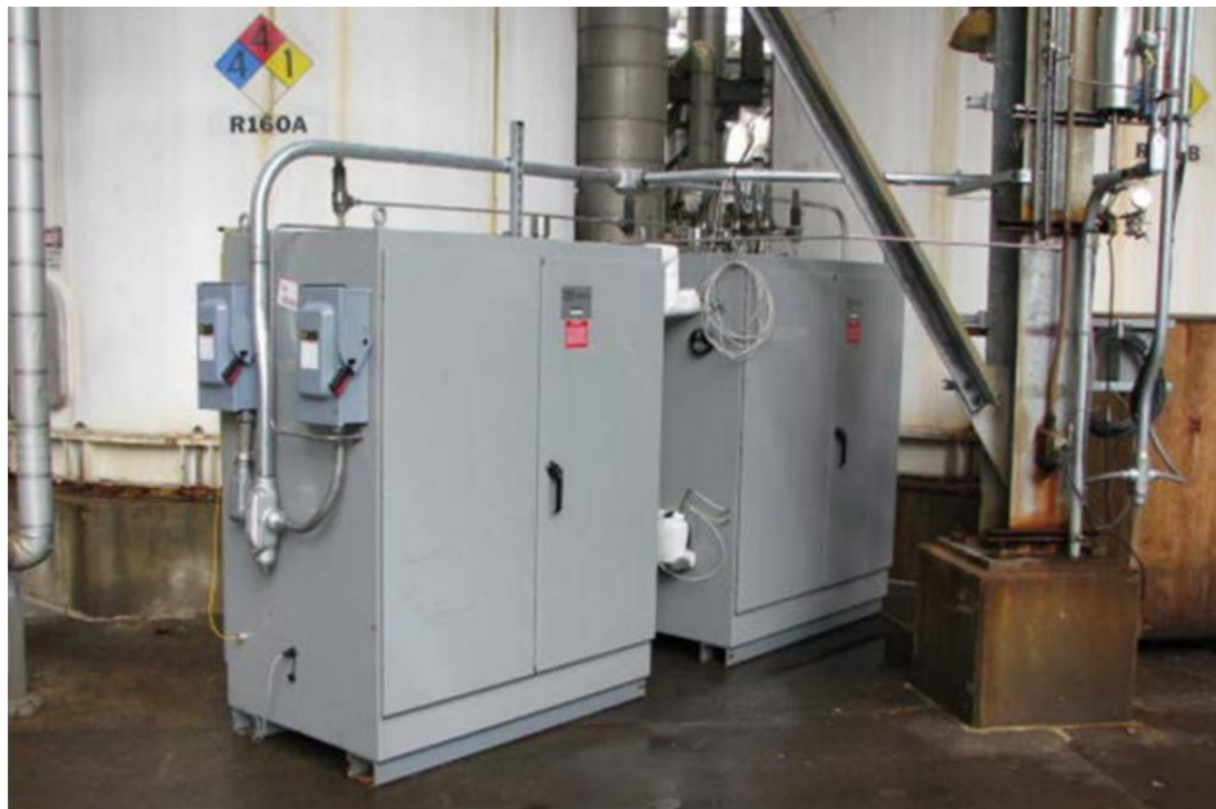
Figure 5-17 Field test units installed at Wabash River IGCC
