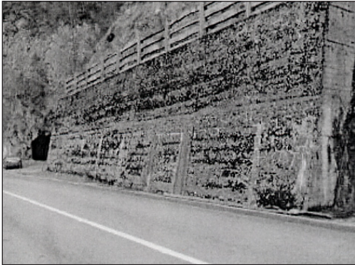
Figure 3. Retaining walls often border close to the roadway, blocking animal movements between habitats on either side of the road.
