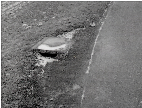
Figure 5. This gully traps many amphibians each year, even though there is no curbstone guiding the animals to the entrance. The animals climb into the opening, expecting a humid shelter.
