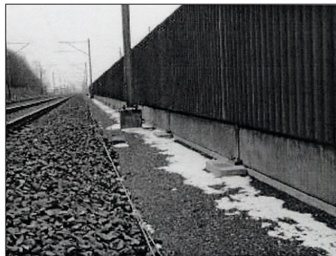
Figure 8. Noise barrier along a railroad line.
