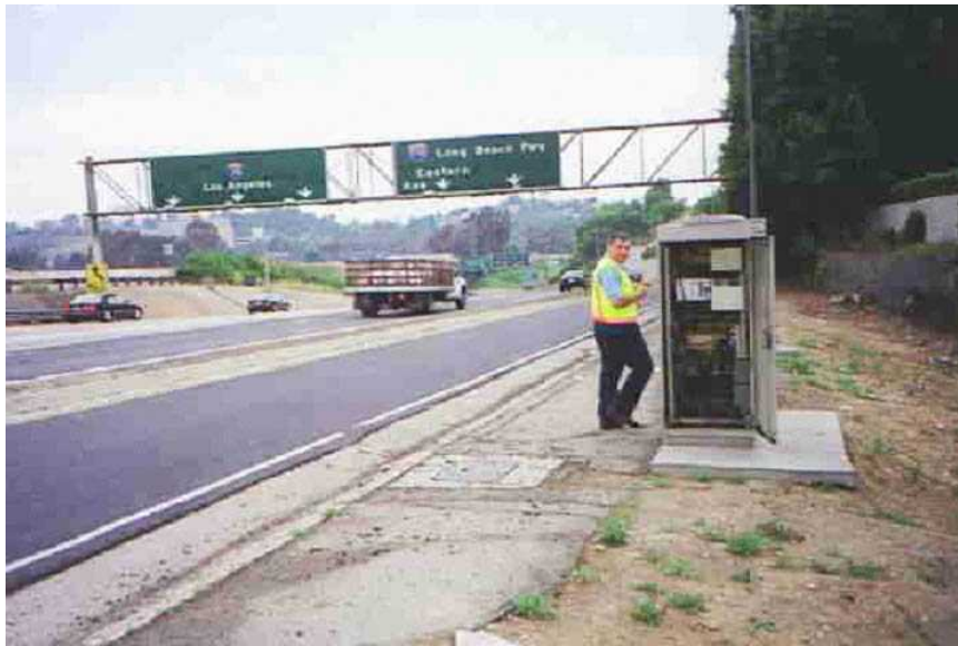
Figure 4.4: Cabinet location next to freeway.
