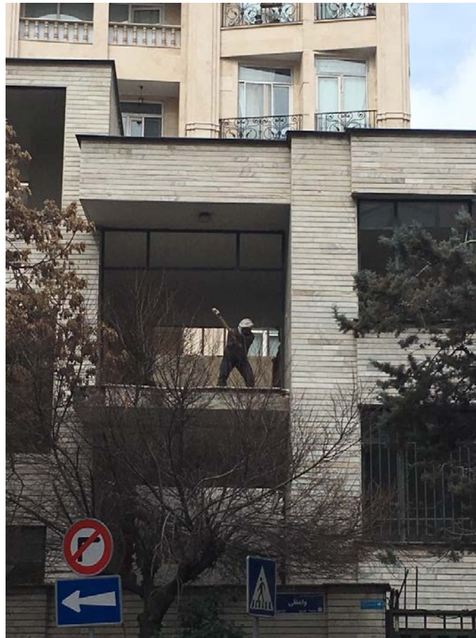
Figure 2.2: A building being demolished with a pickax in northern Tehran. Source: photo taken by author, 2018
