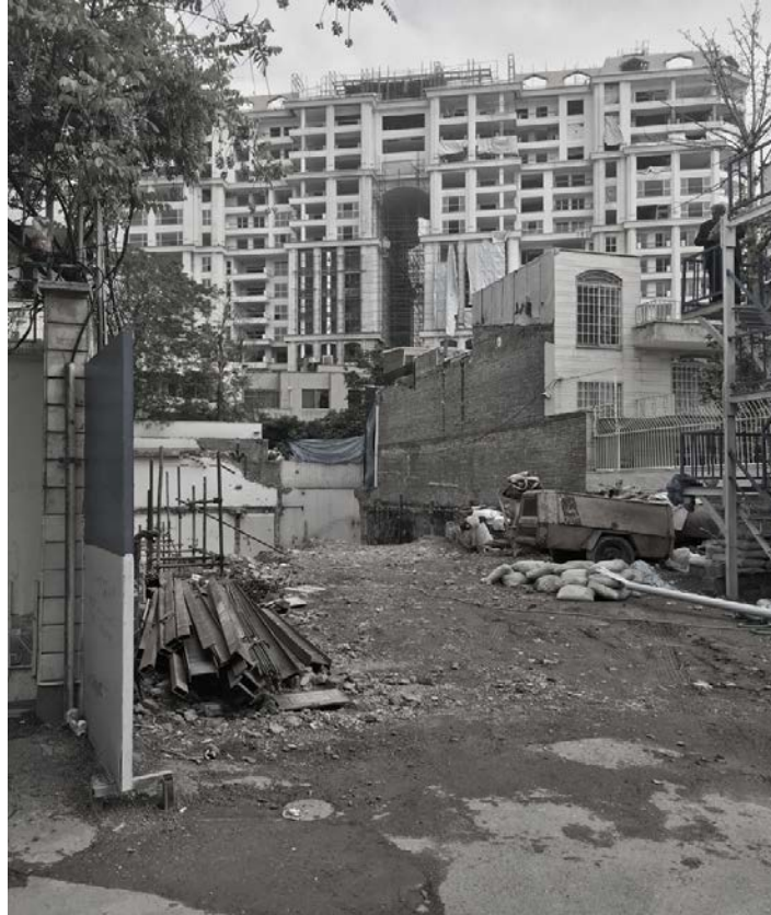
Figure 1.3: A site of construction in a narrow alley in northern Tehran. Source: photo taken by author, 2018
