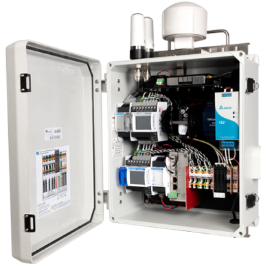
Figure 5: The \mu PMU sensor holds the promise of increased distribution network visibility. The white “mushroom” on top of the device box is an antenna for receiving the GPS clock signal.
