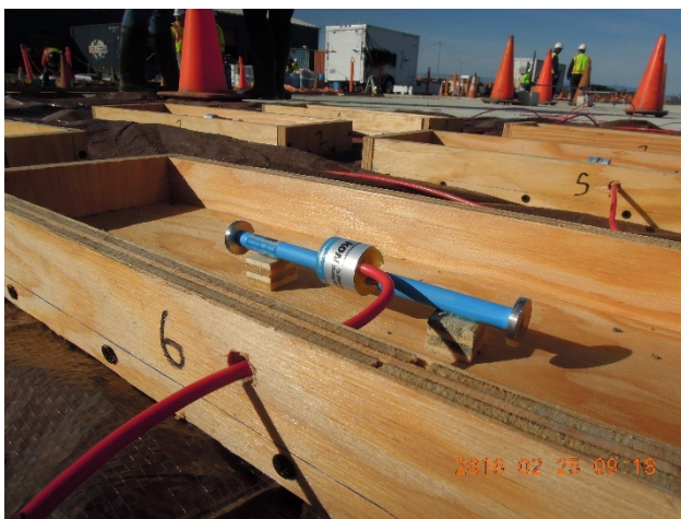
VWSG inside the mold
