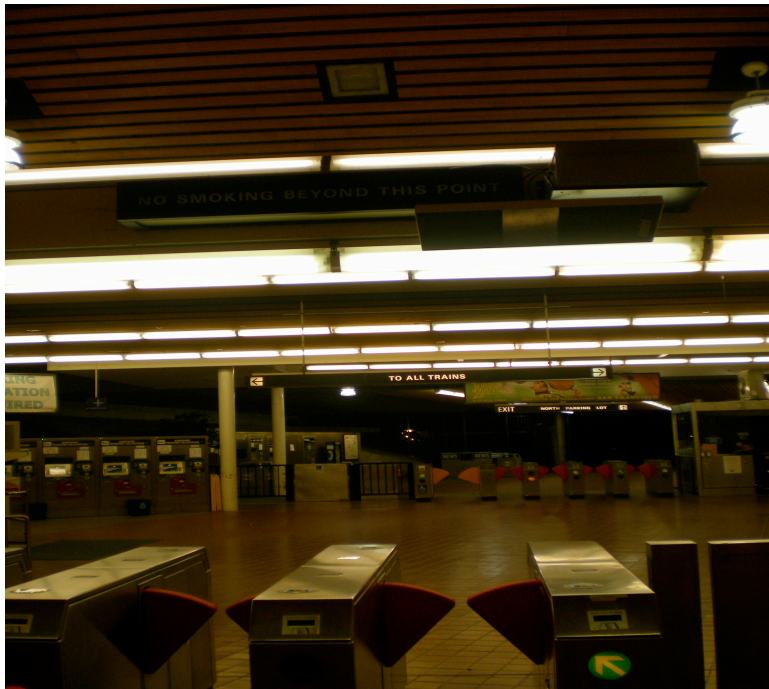
Figure 6. RFID Reader At the Entrance of BART Lafayette Station (Reader and Its Antenna are mounted on top of the entrance near the ceiling)
