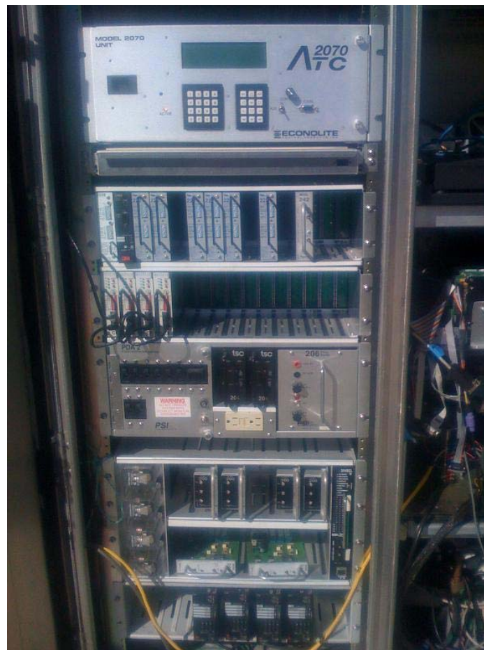
Figure 3.2: 2070 traffic controller at RFS Intelligent Intersection
