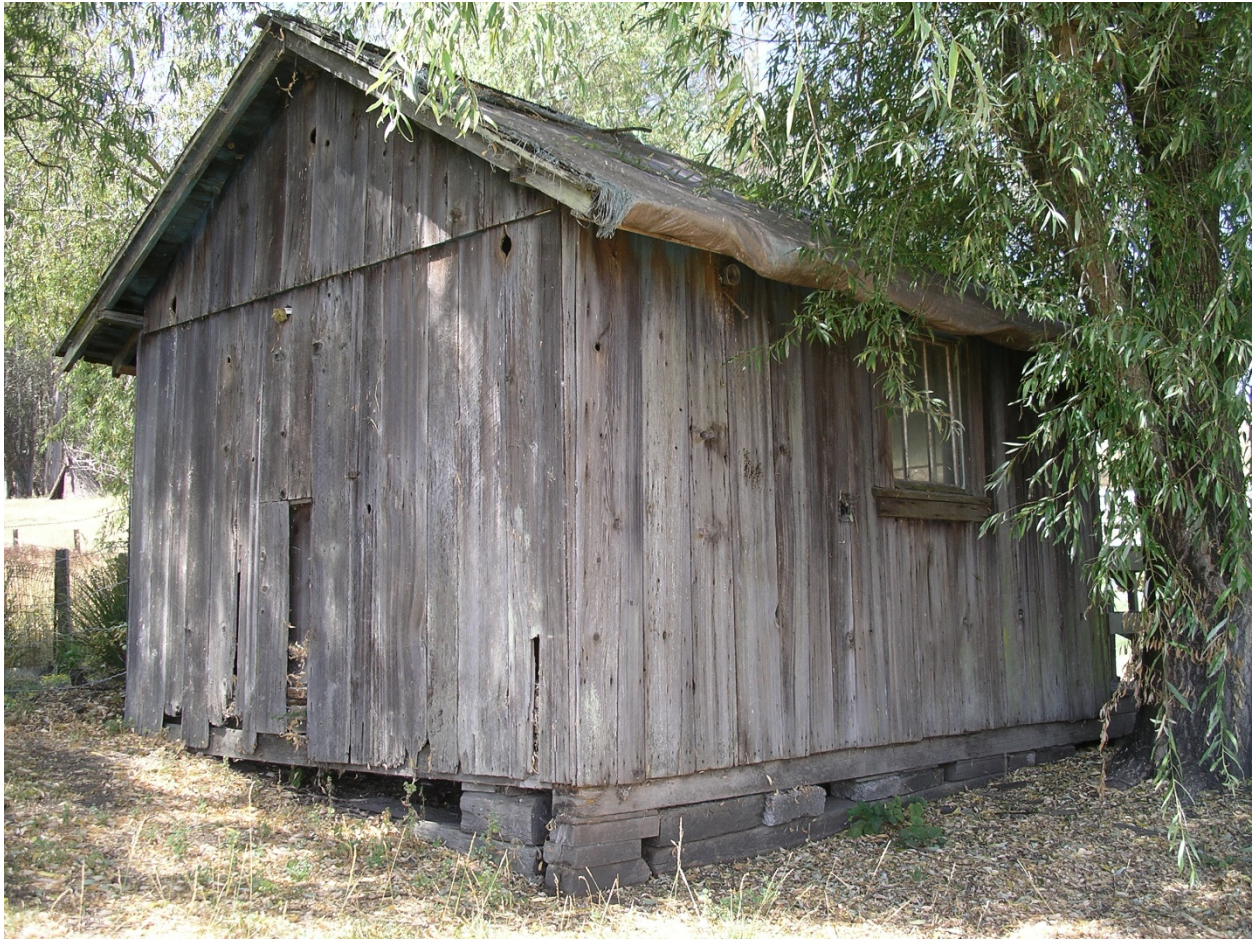
Figure 4.7. Image of a wooden house/shed on sleds that could be pulled by a team of horses to different parts of the property and propped up in a level position with additional blocks and beams.
