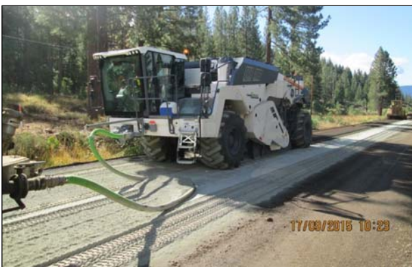
Figure 3.18: PLU147: Water pipe dragging on cement.
