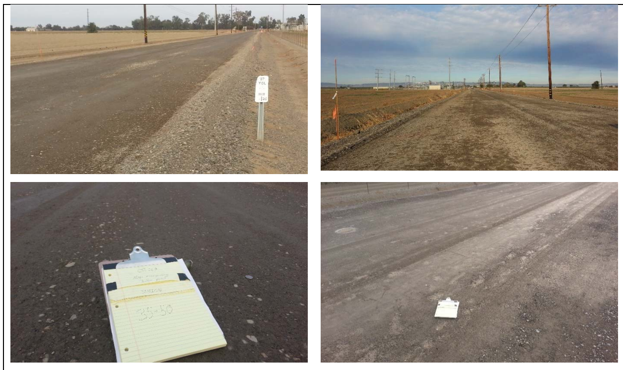
Figure 3.32: CR27: Photographs showing wet surface.
