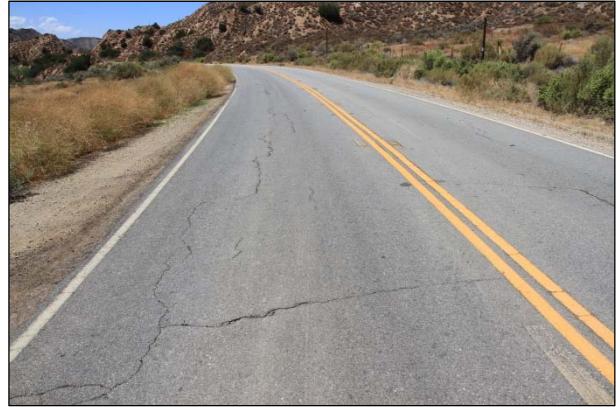
Figure 2.4: Block crack progression.
