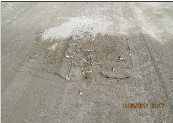
Figure 3.6: CR32B: Wet, soft location after final compaction.
