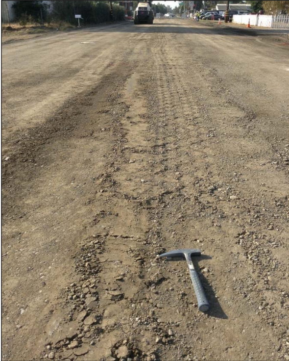
Figure 3.13: CR99: Delamination after microcracking.
