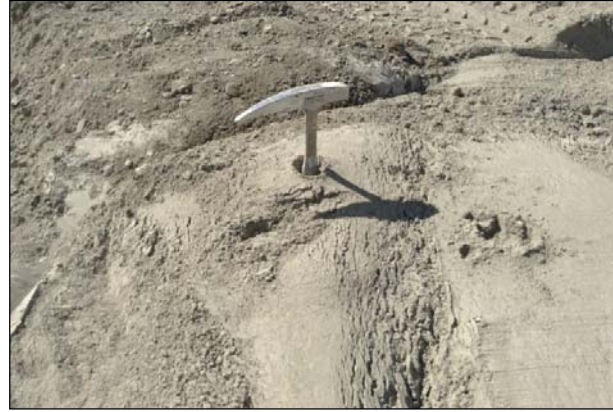
Figure 3.21: PLU147: Depth of cement mound due to dragging of hose ( \pm 200 mm).
