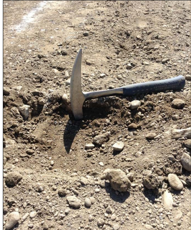
Figure 3.14: CR99: Depth of delaminated material (50 mm [2 in.]).
