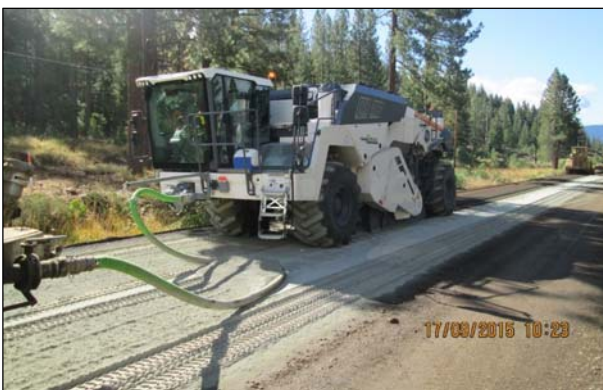
Figure 3.18: PLU147: Water pipe dragging on cement.
