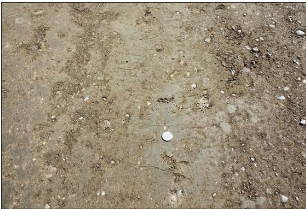
Figure 3.2: CR32B: Transverse cracking after microcracking.
