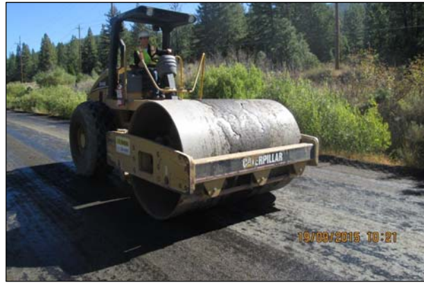
Figure 3.17: PLU147: Prime coat stripping from FDR-PC layer during microcracking.
