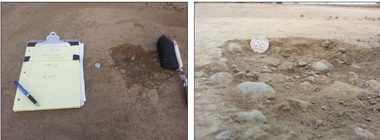
Figure 3.12: CR27: Distressed surface of FDR-PC layer after microcracking near start of project.
