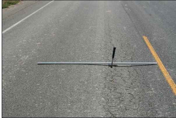
Figure 2.7: Rutting caused by water ingress through cracks into the base.
