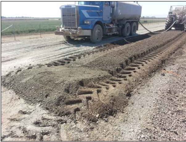
Figure 3.23: End of pulverizer pass with no accumulated cement visible.
