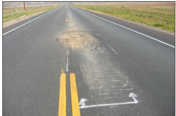
Figure 2.6: Pumping through fatigue cracking.
