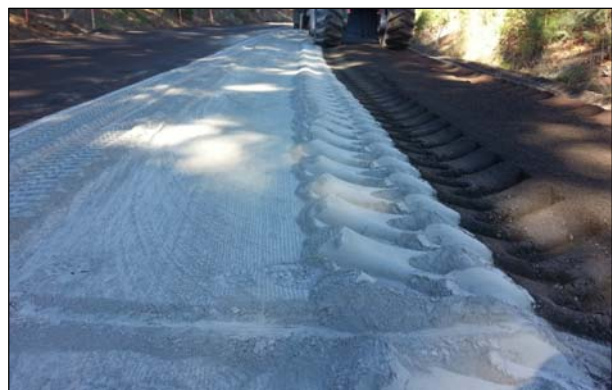
Figure 3.19: PLU147: Accumulation of displaced cement in pulverizer wheel track.
