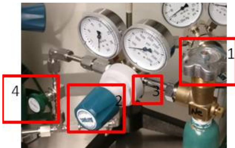
Figure B.7: Example of the 4 valves on each gas cylinder (1: Bottle valve, 2: pressure regulator, 3: regulator valve, 4: pipe valve)
