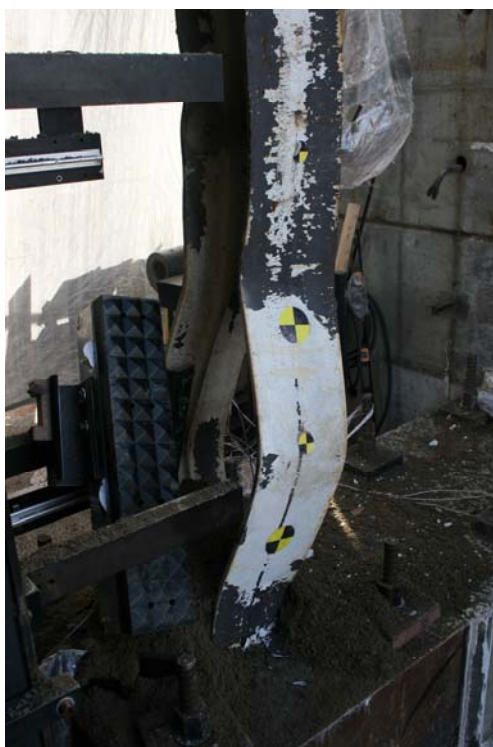
Figure 5.64: Test WA06 Column Base Post-Test
