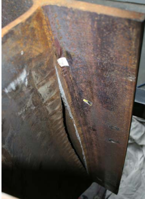
Figure 6.43: Crack Propagation from 25 m/s Test
