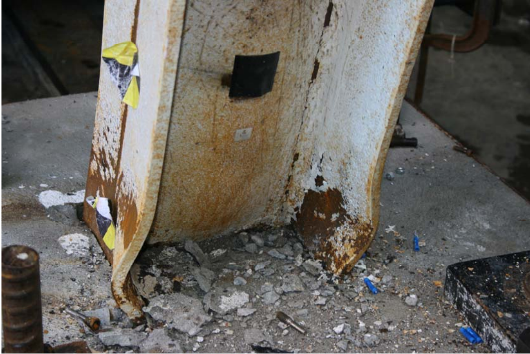
Figure 5.57: Test WA05 Base Buckling (Non-Impact Side)
