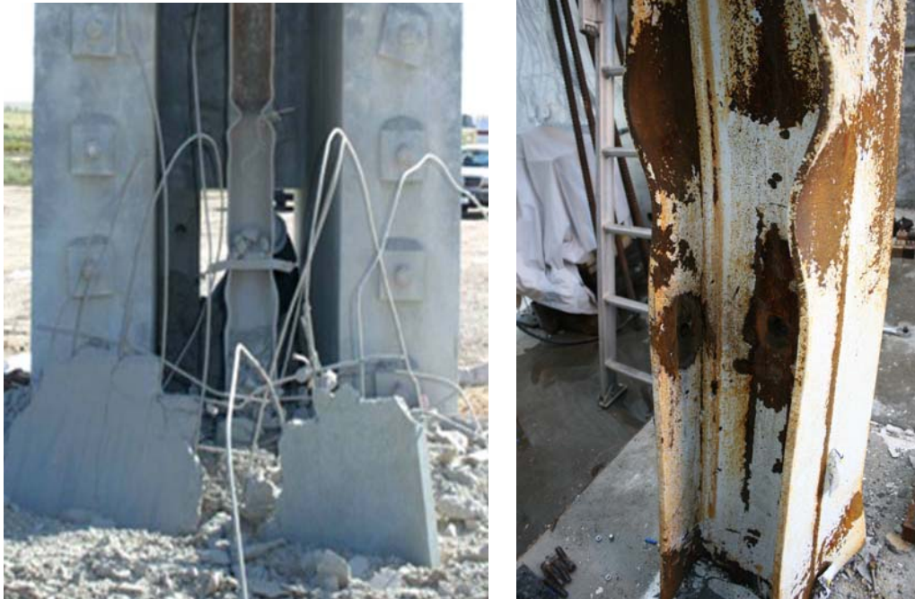
Figure 5.71: Field Test 8 (left) and WA05 (right) Localized Flange Behavior Comparison
