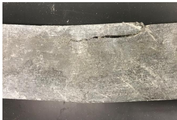
Figure 108: Close-up front view of final failure region in casted prismatic beam (Specimen CL PTV-7) with same total volume as topology-optimized beams and with additional horizontal constraints at supports.
