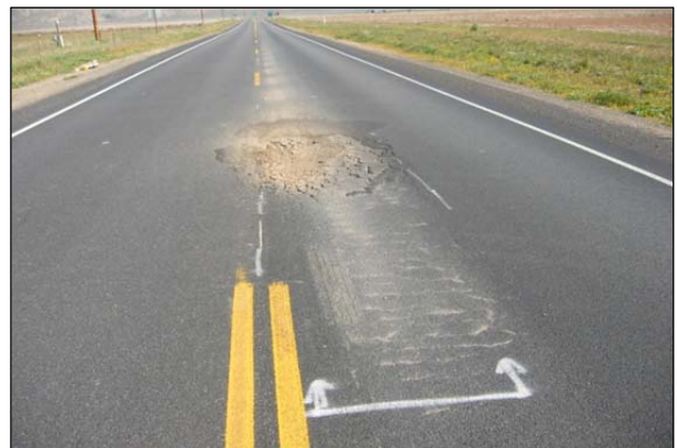
Figure 2.6: Pumping through fatigue cracking.
