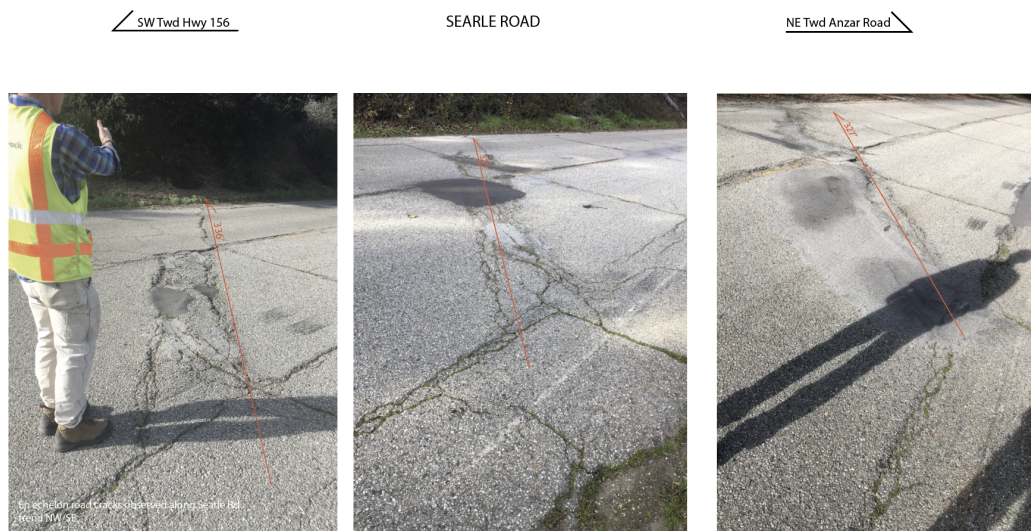
Figure 14. Three en echelon cracks located along Searle Road trend NW/SE showing repeated road repair.
