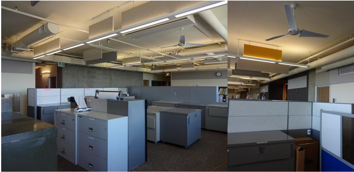
Left: Open office space with radiant ceiling, ceiling fans and overhead mixing diffusers for ventilation only. Right: Ceiling fan over open office cubicle.
