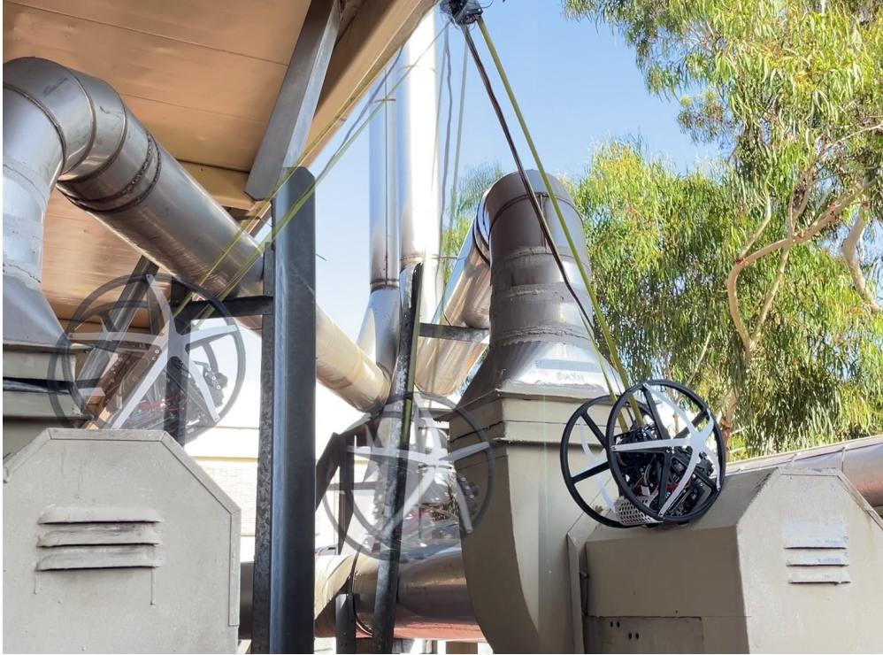
Figure 4.29: Overlaid screenshots of EEWOC swinging between two surfaces on HVAC equipment.
