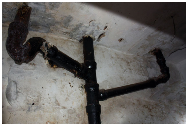
Figure 3. Wastewater pipes in Block C2 of Quang Trung housing, Vinh City, Vietnam, 2011. Photo by C. Schwenkel.
