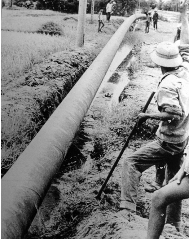
Figure 4. Laying a water supply line from the central water plant to Quang Trung housing, Vinh City, Vietnam, 1975. Courtesy of the Nghệ An Provincial Museum.
