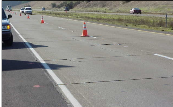
Figure 2.7: Example of faulting and transverse and corner cracks on concrete pavement.
