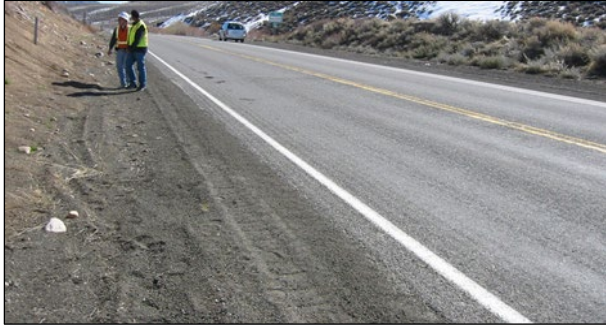
Figure 3.32: Cut slope with no side drain.
