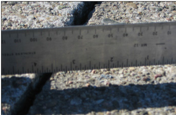
Figure 3.18: Faulting on jointed plain concrete slabs.
