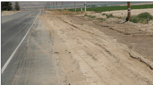
Figure 3.30: Irrigation water sprays onto the road.
