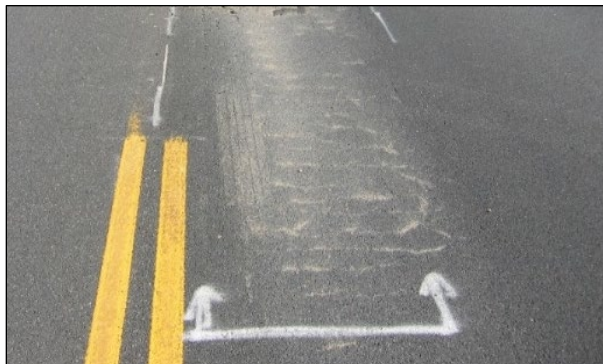
Figure 3.11: Pumping of fines from underlying unbound layers through fatigue cracks.
