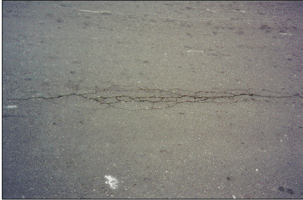
Figure 3.1: Initial fatigue cracking in wheelpath.
