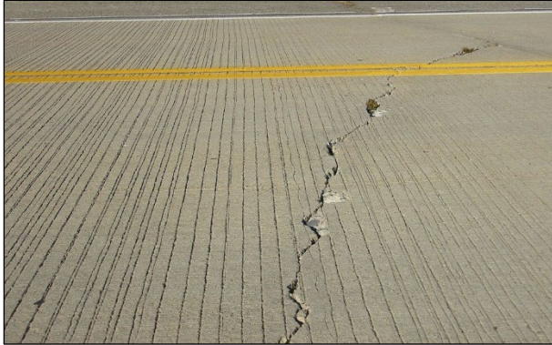
Figure 3.16: Transverse crack with spalling on jointed plain concrete slabs.
