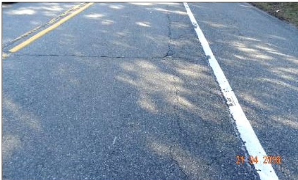
Figure 3.7: Reflected cracking from underlying jointed plain concrete slabs.
