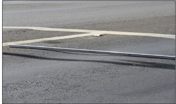
Figure 3.10: Rutting in unbound layers (no humps).
