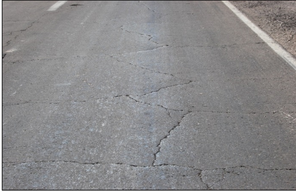
Figure 3.5: Oxidative-aging cracking in block pattern.
