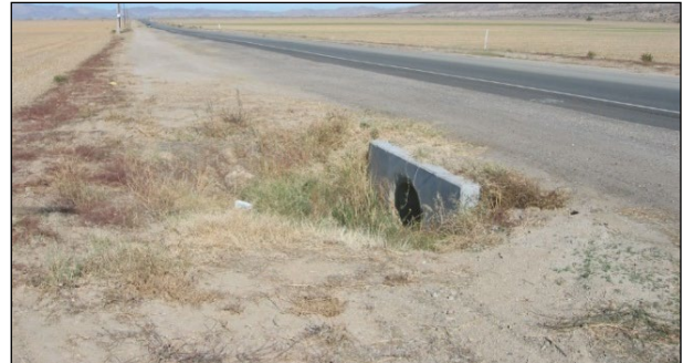
Figure 3.27: Blocked side drain and culvert.
