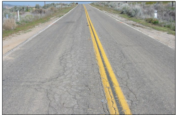
Figure 2.4: Example of Alligator B cracking.
