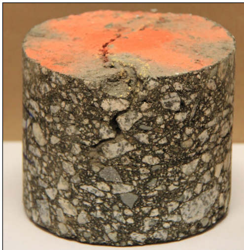
Figure 3.44: Partial-depth top-down crack (caused by low temperatures).
