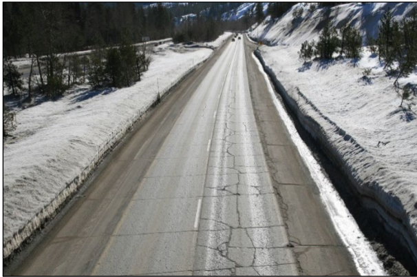
Figure 3.14: Jointed plain concrete truck lane with shattered slabs.
