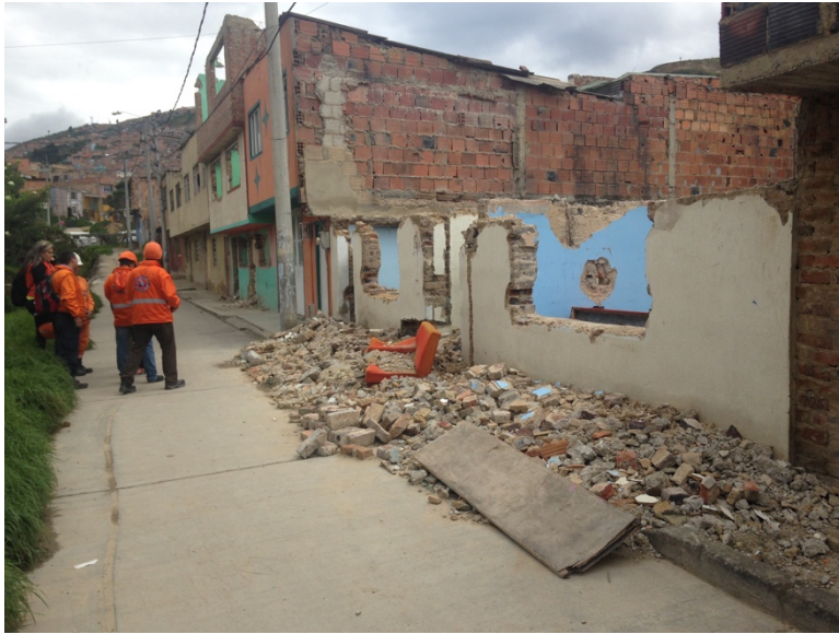
Picture 2. Civil Defense team inspecting a home demolished by IDIGER in Ciudad Bolivar
