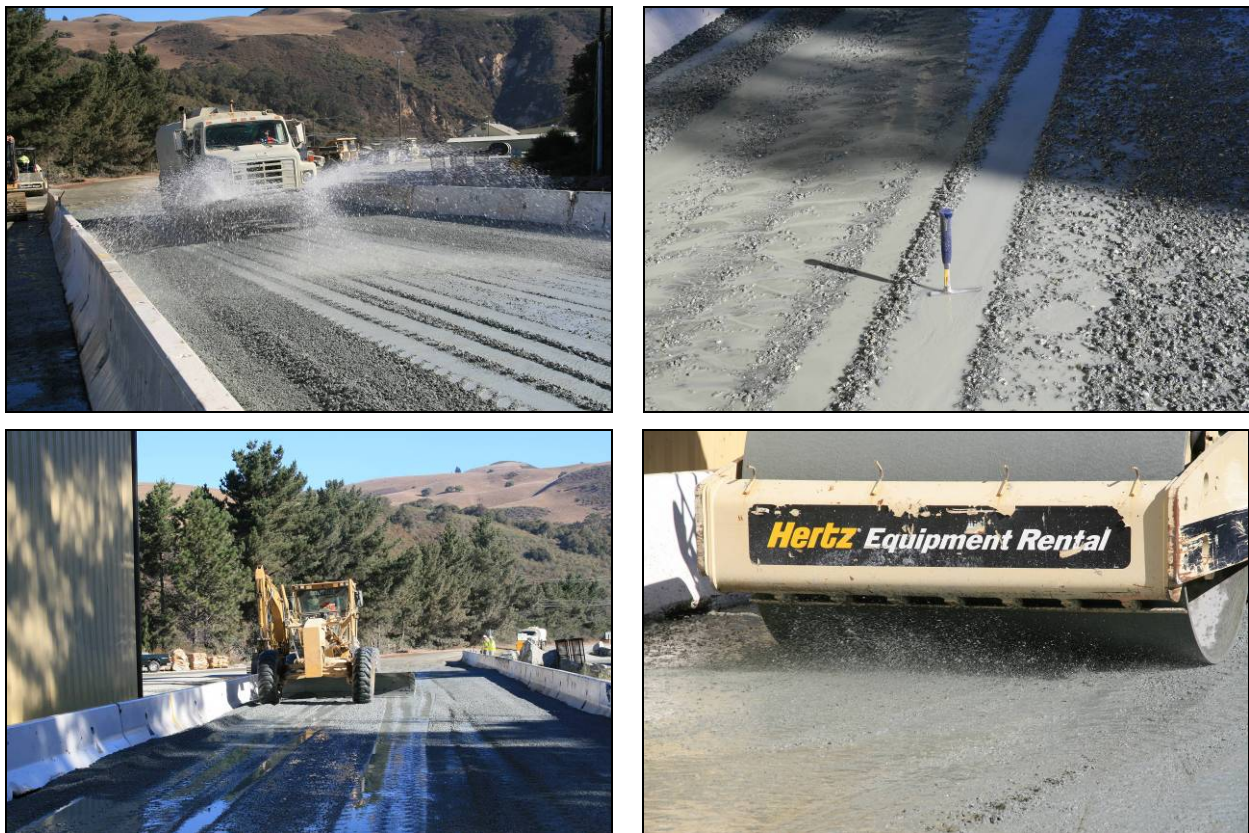
Figure 2.9: Overwatering during base-course construction.
