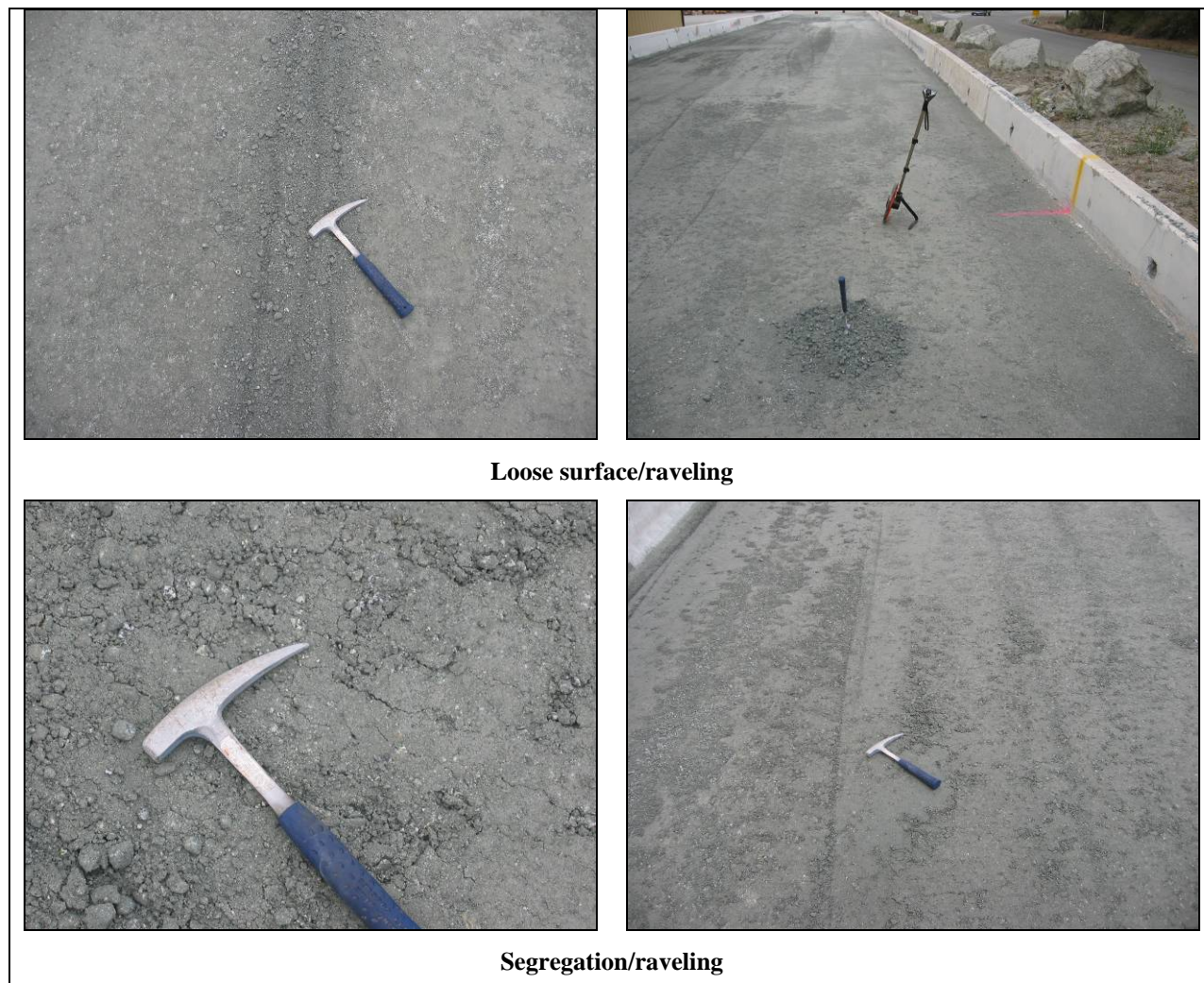
Figure 2.12: Isolated areas of distress on the base-course.
