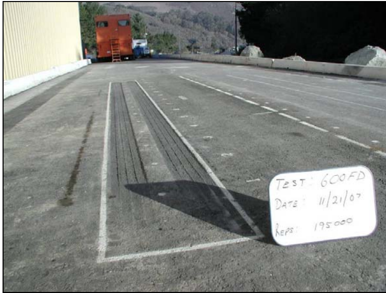
Figure 4.11: 600FD: Section photograph at test completion.
