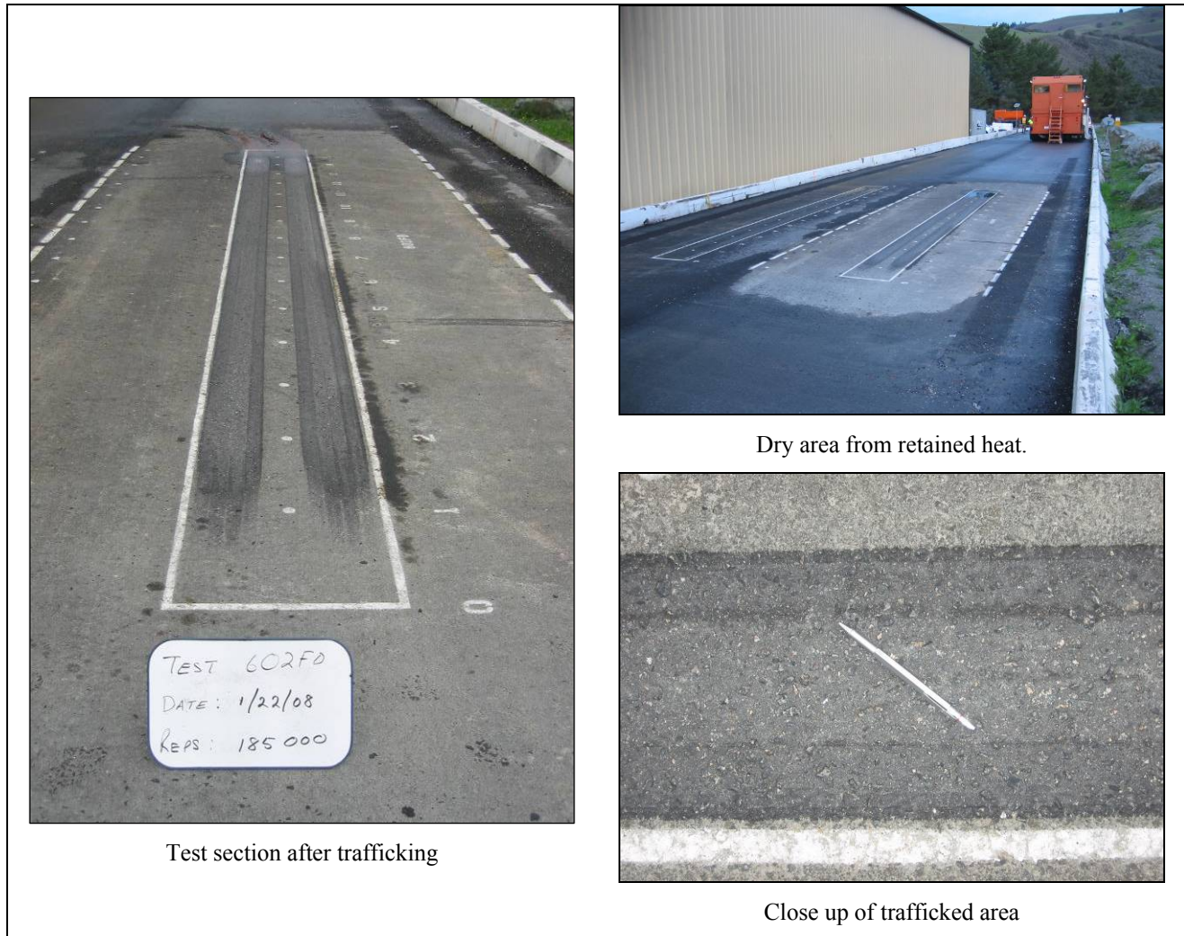
Figure 4.28: 602FD: Section photographs at test completion.
