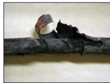
Failed cable after flashover.
