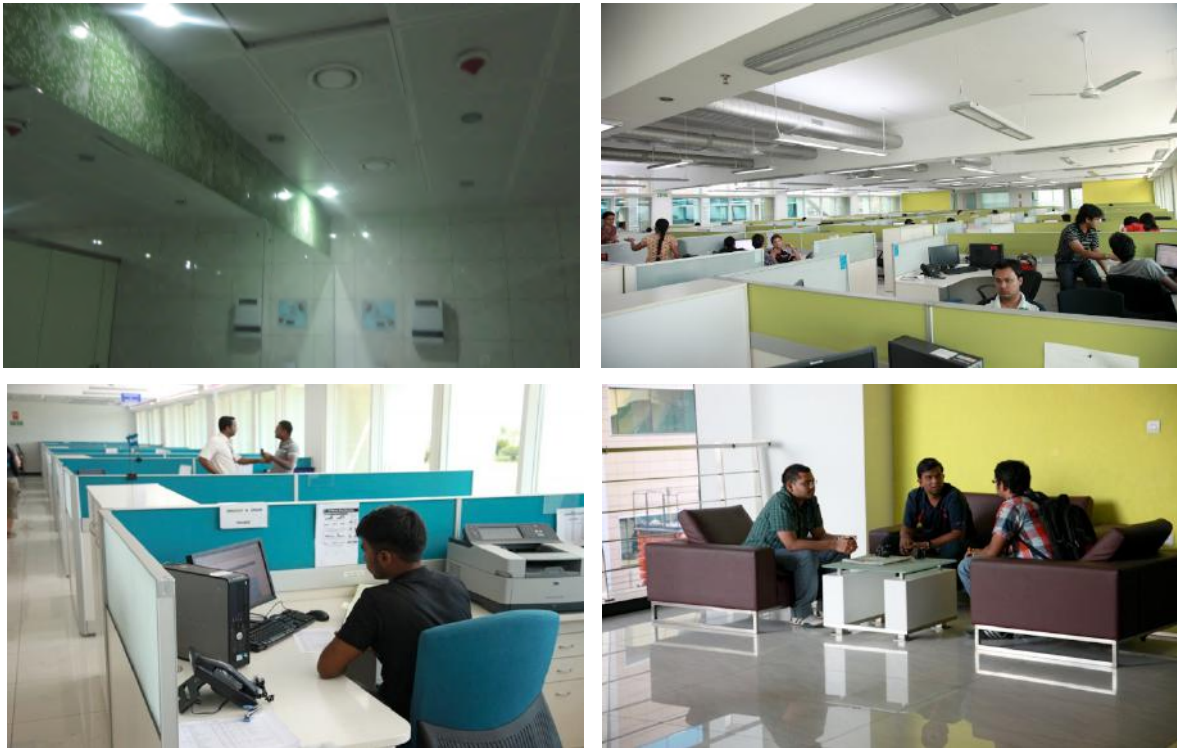
Figures: Infosys, Pocharam. Top left: occupancy sensors in the restrooms. Top right: T5s and LED down lights are used. Bottom left and right: The amount of daylighting in the office spaces and lobbies has minimized the requirement for artificial lighting substantially (photos: Infosys Green Initiatives Team).
