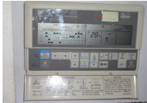
Figure: Flexible Setpoint Management (Photo: Facilities Team, Sears Holdings India)
