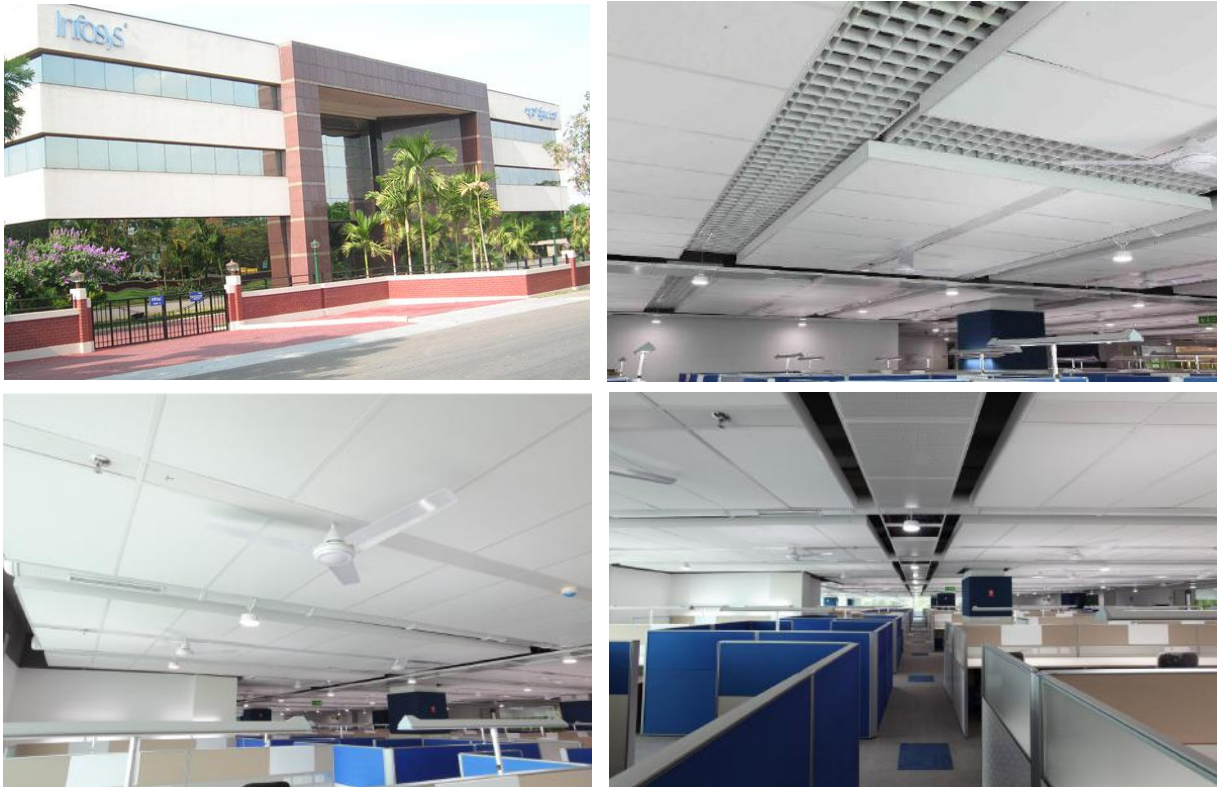
Figure: Radiant panels and ceiling fans at the MC1 building at Infosys, Bangalore. (Source: Infosys, Uponor)
