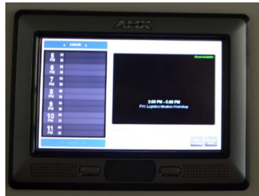
Figure: The calendaring-based lighting controls system in a conference room
