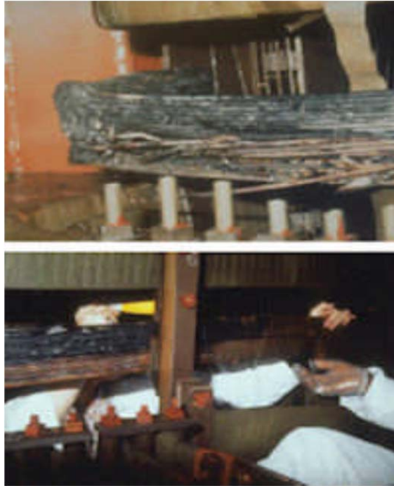
Figure E.1 Salem N.J. Nuclear Plant GSU Transformer Damage
